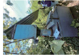
Figure 16: Incinerator 1 – not functional
