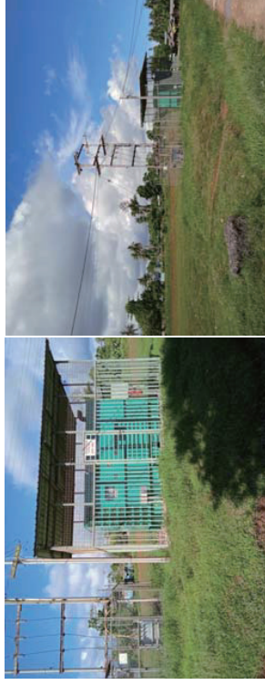
Photo 13 and 14. Transformer and the standby generator
