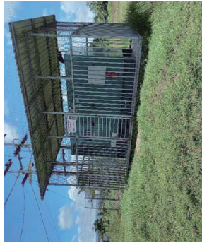
Figure 11: Backup diesel generator
