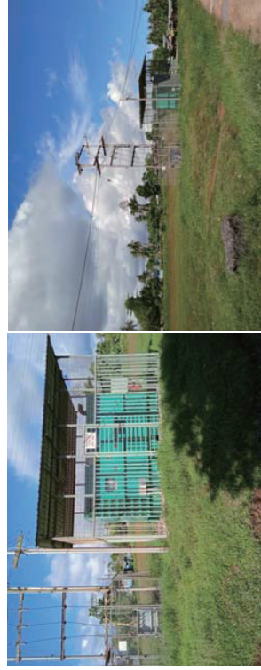
Photo 13 and 14. Transformer and the standby generator
