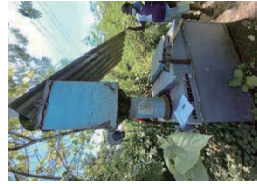
Figure 16: Incinerator 1 – not functional
