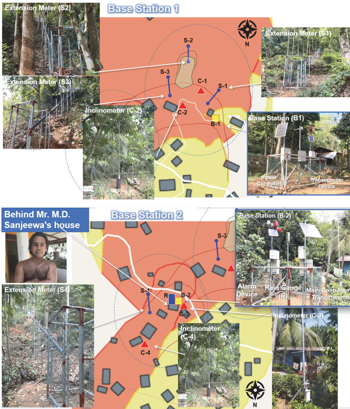
Figure 37: Location and image of installed extensometers and multi-point inclinometers in Udapotha (Base Station 1 & 2)
