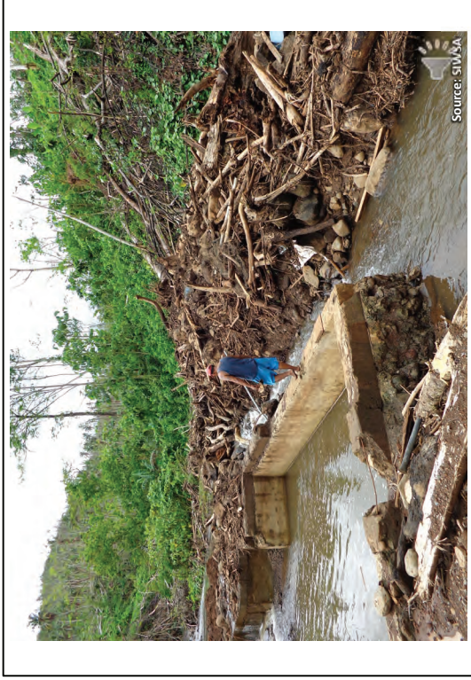
This photo shows the effects of Cyclone Gita on Letogo scheme's intake. The debris that washed into the intake was cleared away by the villagers.
