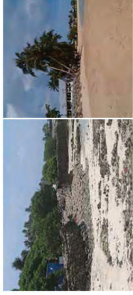
Figure 3-4 A stacked coral block wall in Kiribati collapses, forming a "Dynamically Stable Revetment" (left) and sand replenishment at Manase, Samoa (right)
