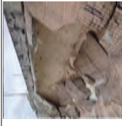
Damage of infrastructure (coastal dike)
