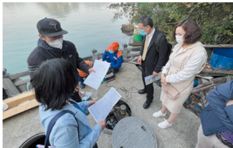
Viet Nam: JICA experts being briefed on how Japan-made septic tanks are operated and maintained on Ti Top Island at the World Heritage Site of Ha Long Bay
