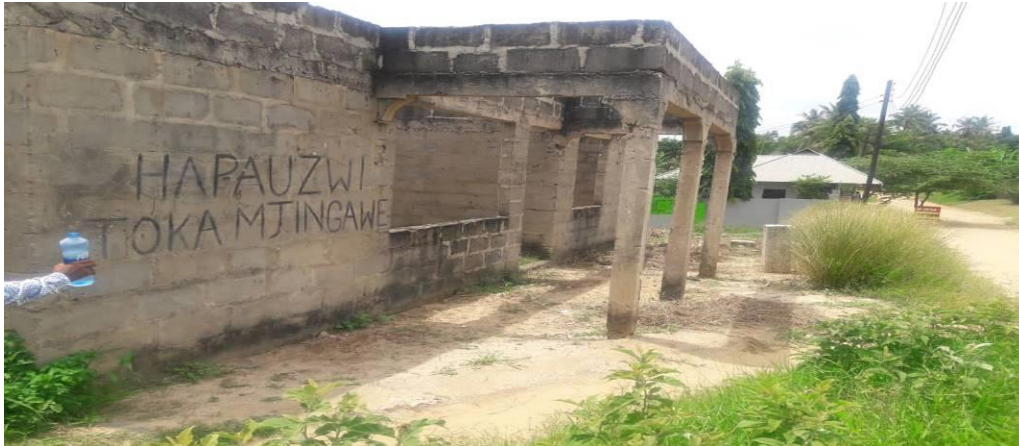
Photo 3: Incomplete structure at Kilungule B in Kimara ward
