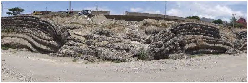
3.8km (Right bank): Gabion mattress is collapsed and traffic of a road on the bank is affected.
