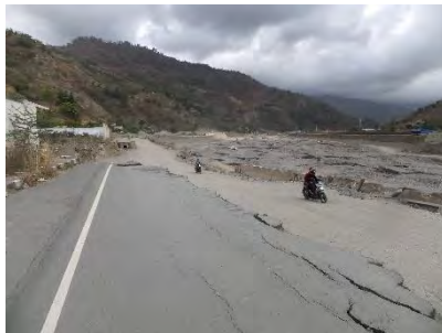
5.5km (R): Retaining wall is dropped and a road on the bank is washed out.
