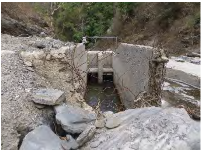
Intake: Falling rocks from the left slope devastated the wall, wing, etc.
