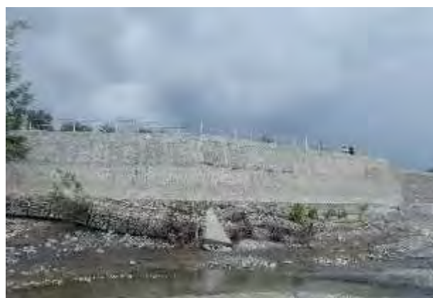
Figure 3.4-6 Scouring of stone masonry wall
