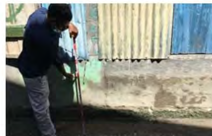
Inundation trace of about 40~50cm
