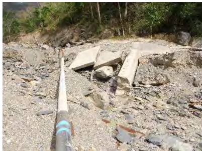
River crossing No.1: Catastrophically damaged except left riverbank
