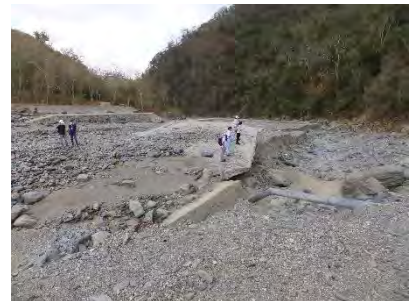
River crossing No.2: Flood flow changed the route beyond the right bank and damaged it.
