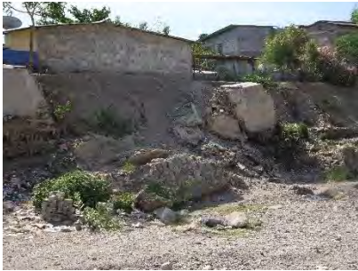
0.9km (Left bank): A part of the damaged section is closed to a runway of the airport.
