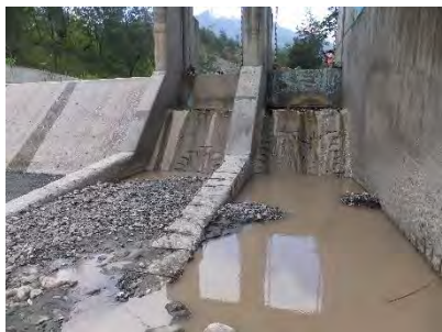
Maliana irrigation: Steel bars of flushing sluice are exposed by wear.
