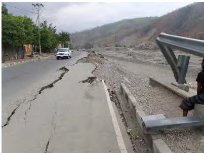
4.1km (R): Retaining wall is collapsed and a part of road is damaged.
