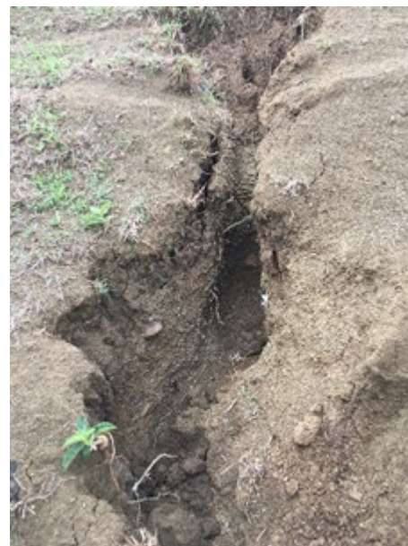
(c) Gully Erosion due to Rain
