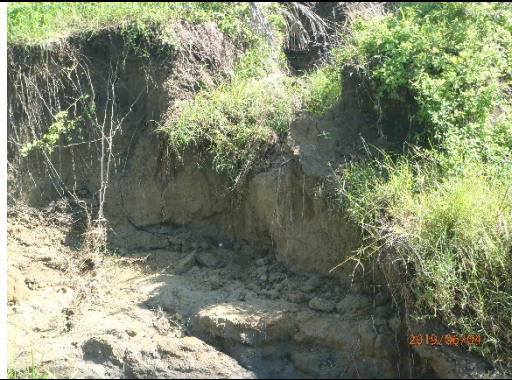
Erosion at Existing Natural Waterway
