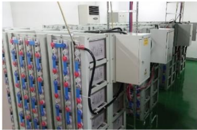
Fig A. Backup Power Supply
