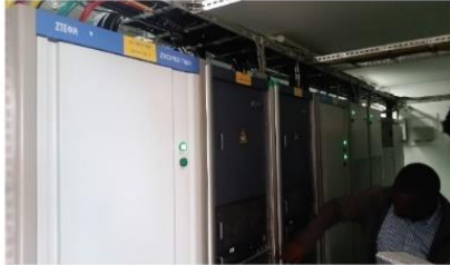
Fig B. Power Management System
