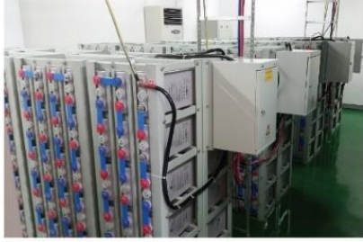
Fig A. Backup Power Supply
