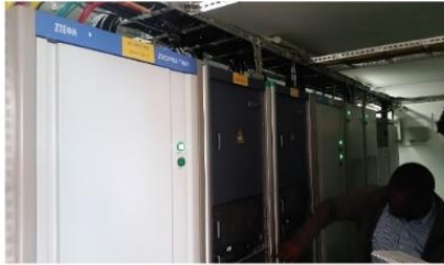
Fig B. Power Management System
