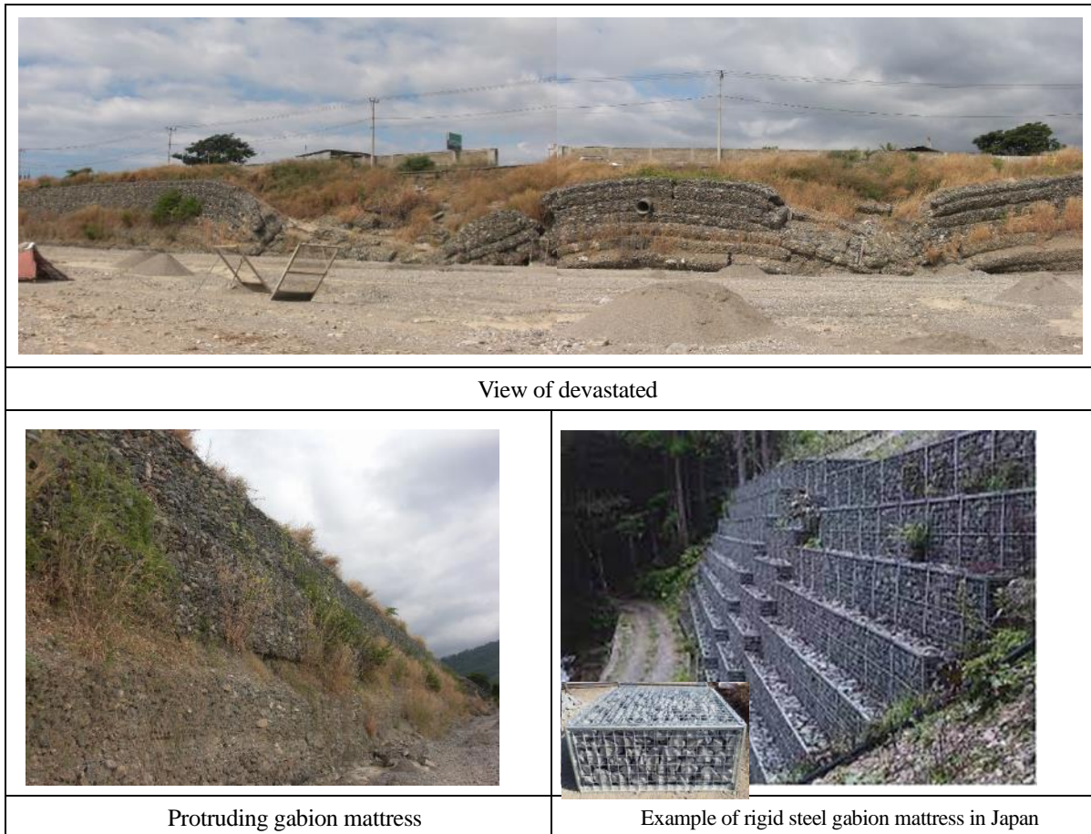
Figure 2-2-1 Situation of damaged R5 revetment
