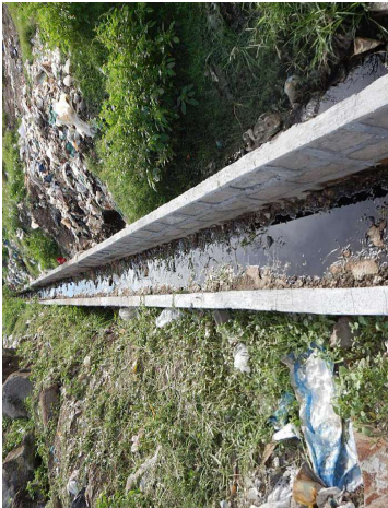
Leachate flowing into perimeter ditches around the landfill
