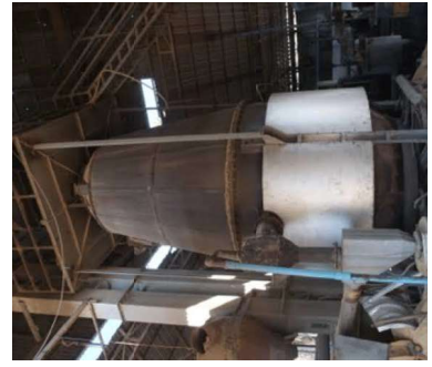
600kW rice husk gasifier
