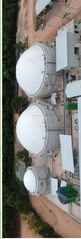
Rayong Biogas Plant
