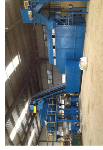
URENCO 11 RPF Facility
