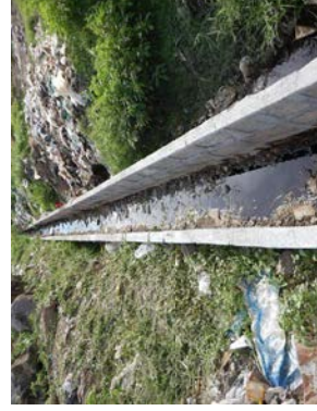
Leachate flowing into the drainage around the landfill
