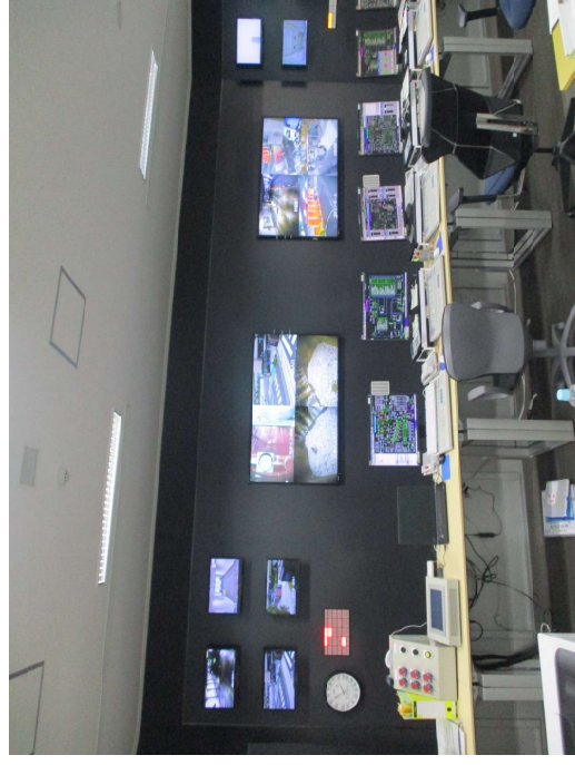
Central Control Room
