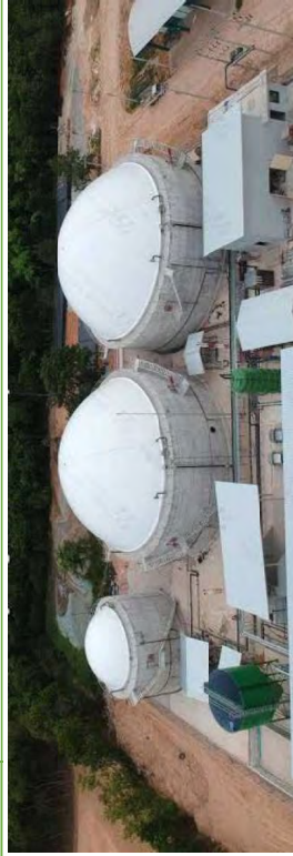
Rayong Biogas Plant
