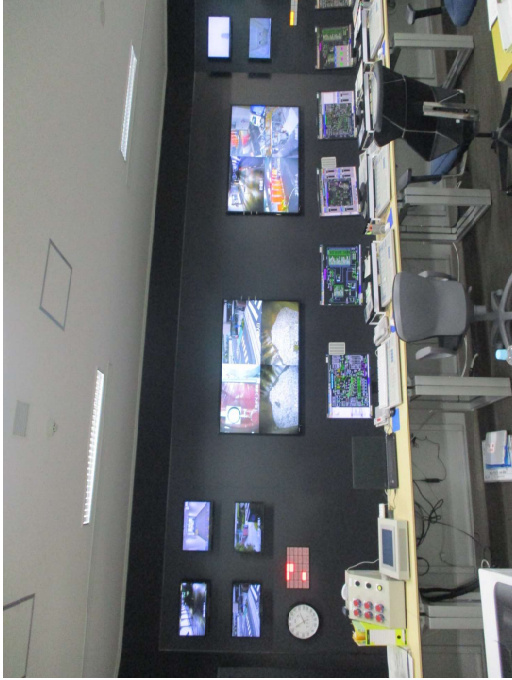
Central Control Room
