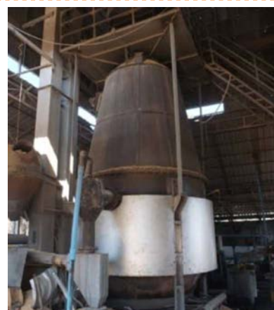
600kW rice husk gasifier
