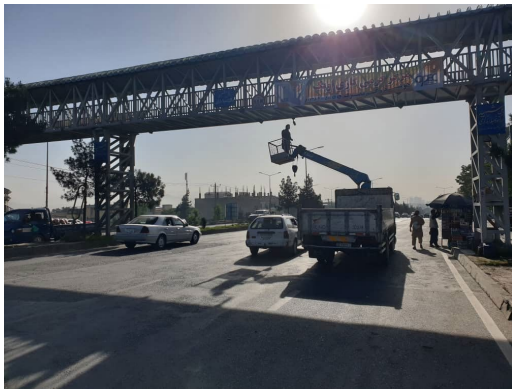
Figure 4: Camera Installation at Baghe Bala Street (S-1)
