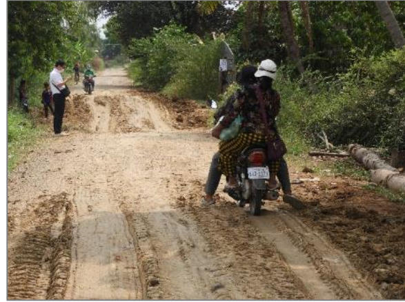
Even several days after the rain, puddles and mud remain in the road sag. It makes drivers difficult to drive motorcycle without slow down. (BTB-4)
