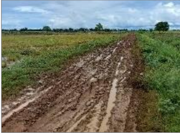
When it rains, the road surface becomes muddy, making vehicles drive very difficult. (BTB-5)
