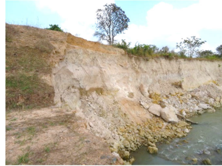
Pic-12 Riverbank collapse (Lum Hach)
