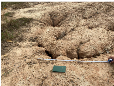
Pic-7 Tunnel erosion (Dragon hole)
