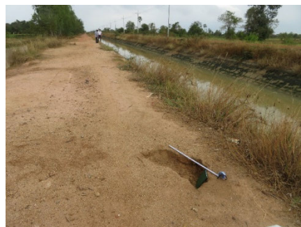
Pic-6 Sinking of maintenance road surface
