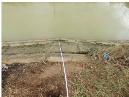
Pic-5 Deformation of concrete blocks
