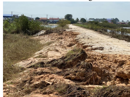
Pic-10 Collapse of the slope
