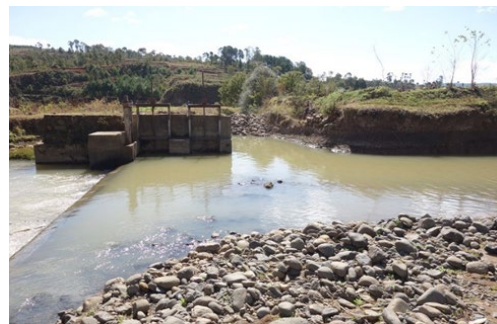
Figure 6.5.4 Partially Collapsed Reinforced Concrete Permanent Weir (Vakinankaratra Region)
