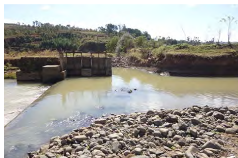
Figure 5 Partially Collapsed Reinforced Concrete Permanent Weir (Vakinankaratra Region)
