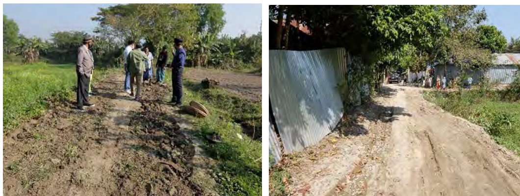
Left: repairing ruts with just putting soils to the ruts without proper compaction works, Right: actual condition of the ruts. Source: JICA Survey Team
