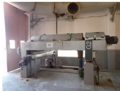
Sludge dehydrator (Sludge treatment facility)
