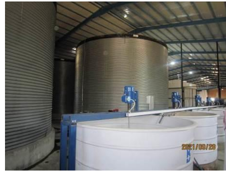
Photo 4-10: Wastewater storage tank in the green house
