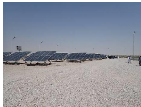
Solar panels (for electric power source of water transmission pump)
