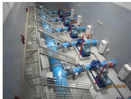
Photo 4-13: Relay pumping station
