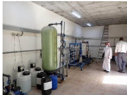
Desalination facility in agricultural test center
