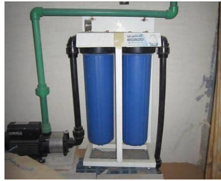
Photo 4-24: RO equipment in far near Bruydah
