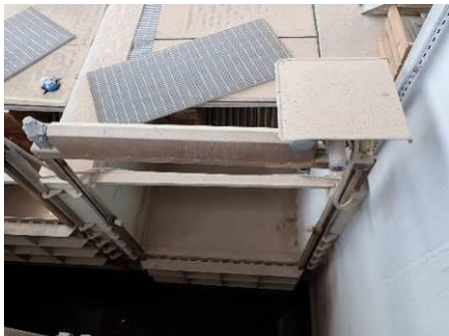
UV disinfection equipment in pump station, under maintenance
