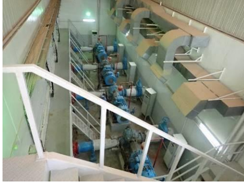
Water transmission pump
