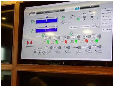
The panel for monitoring operation in the central monitoring room at pump station
