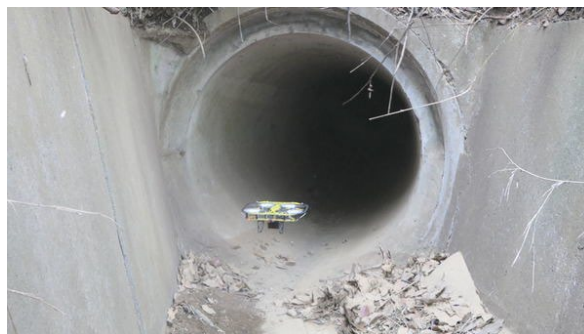
Figure-51 Micro Drone Flying Inside a Pipe
