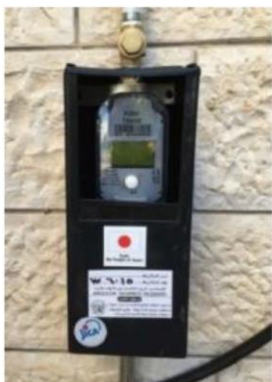
Figure 3 : Photo of a Pre-Paid Water Meter
