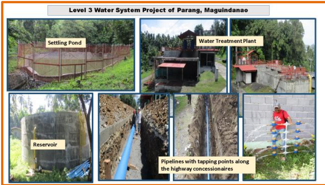
Figure 5.4-16 Photos of the Level 3 Water Supply System in Parang
