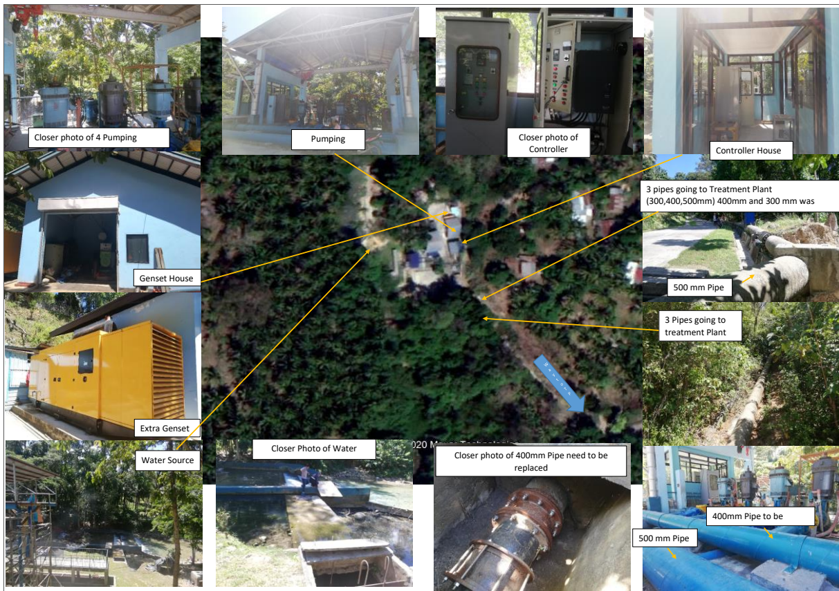
Figure 5.4-8 Photos of Pumping Station in Dimapatoy
