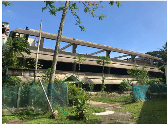
Communications Building that burned down
