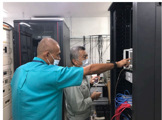
Server at Laucala campus in Fiji
