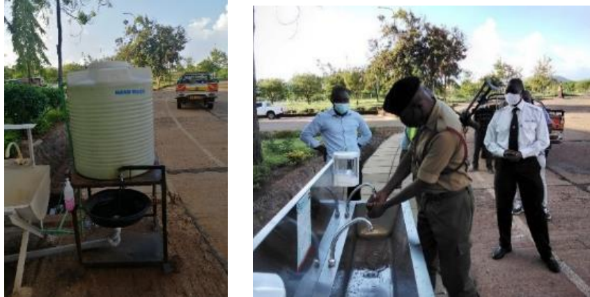
Older handwashing station (left); the newly installed handwashing station (right) at Taveta BP
