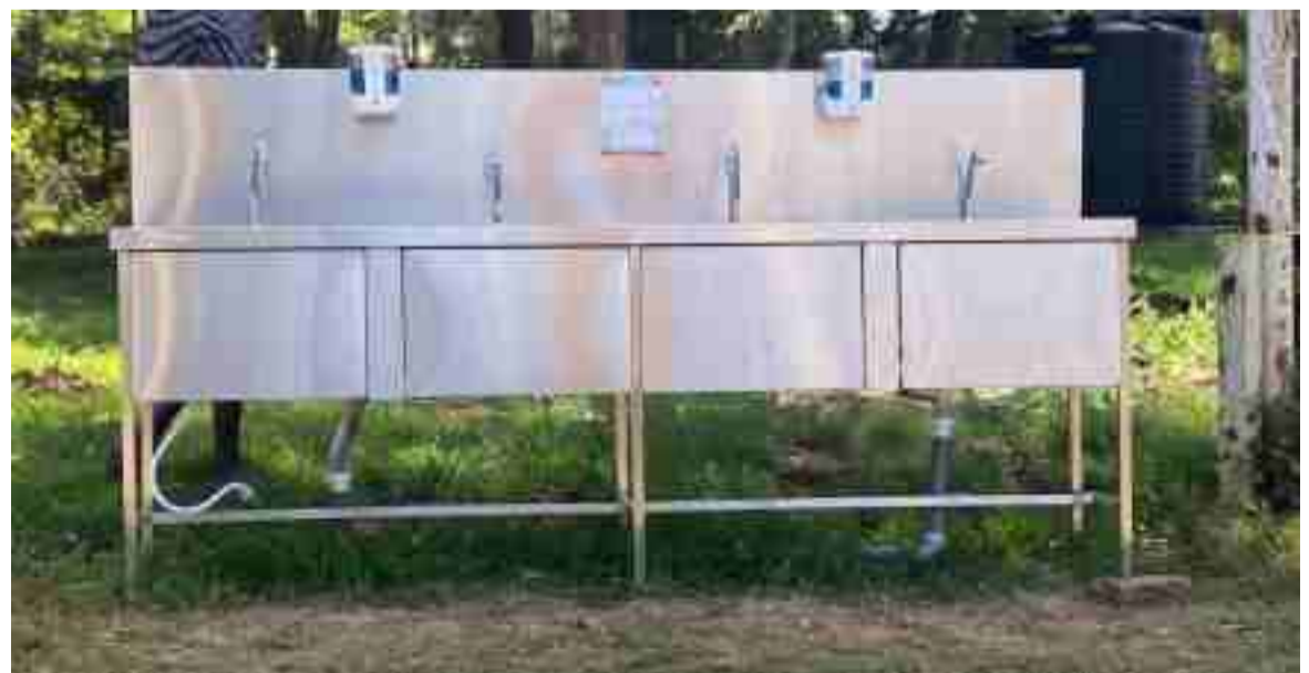
Hand wash station After
