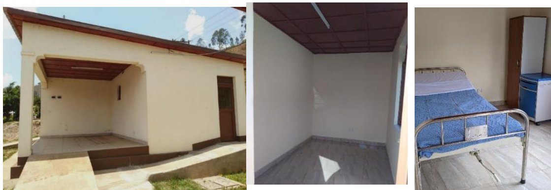
Conditions of the isolation room at Rusumo BP (left);before installation of beds (centre); after installation of beds (right).
