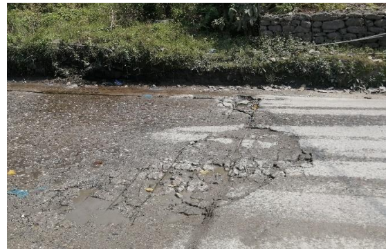
Cracks and Exposed Re-bar
