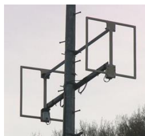
AM Aerial Wire
