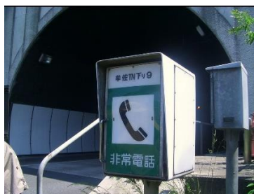
Emergency Telephone at Entrance
