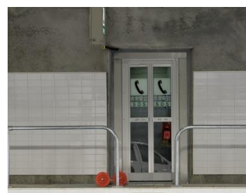
Emergency Telephone Box
