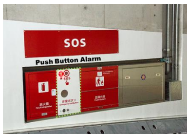
Push Button Alarm with Fire Extinguisher & Fire Hydrant
