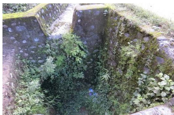
(a) Rainwater Drainage facility
