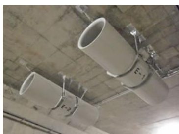
Smoke Removal System (Jet Fan)
