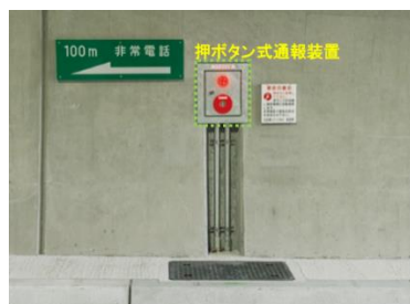
Push Button Alarm
