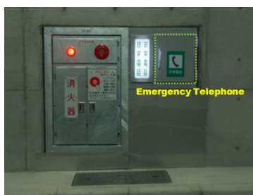
Emergency Telephone on wall
