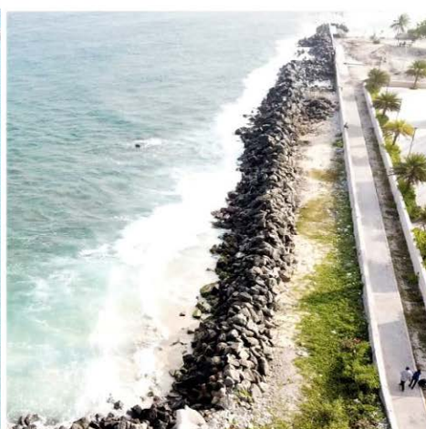
The part where some armor stones were added because of overtopping waves.
