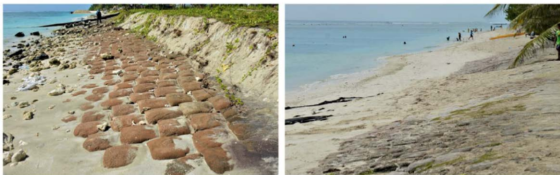
The sandy beach was protected by cement bags, but some areas were eroded and others were covered with sand.
