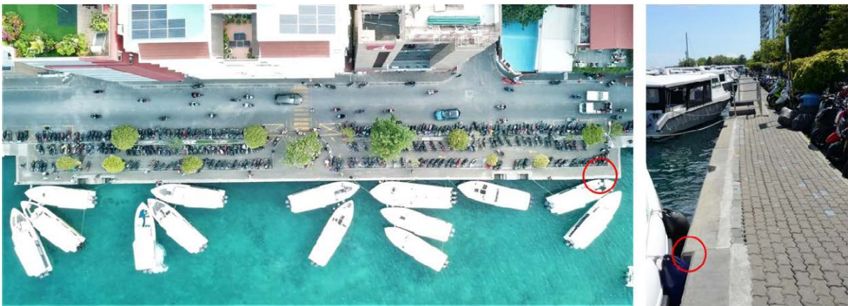
The 95m north seawall that collapsed during the tsunami was restored with a Japan's loan by extending the face line 5m seaward.
