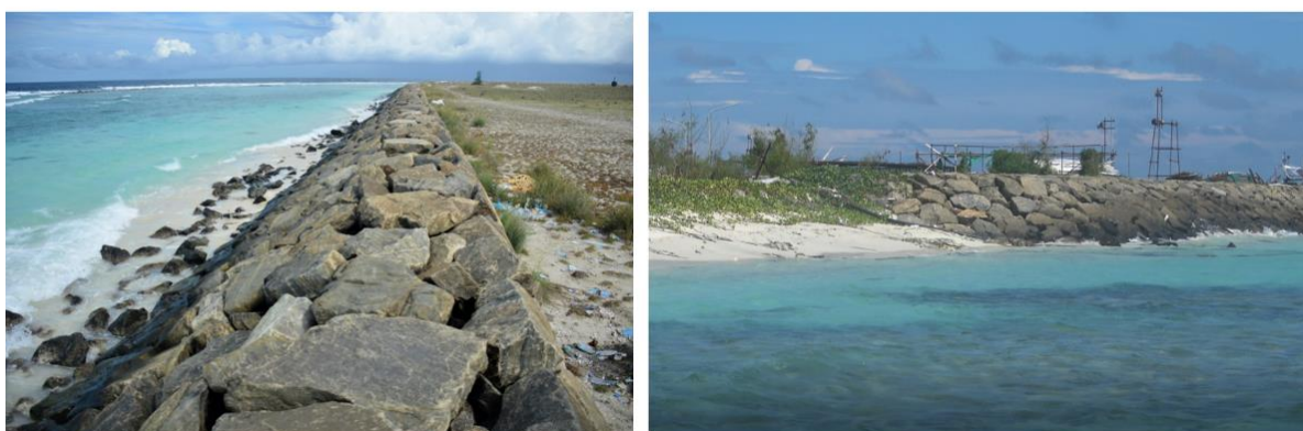
In some places, sand has started to accumulate.
