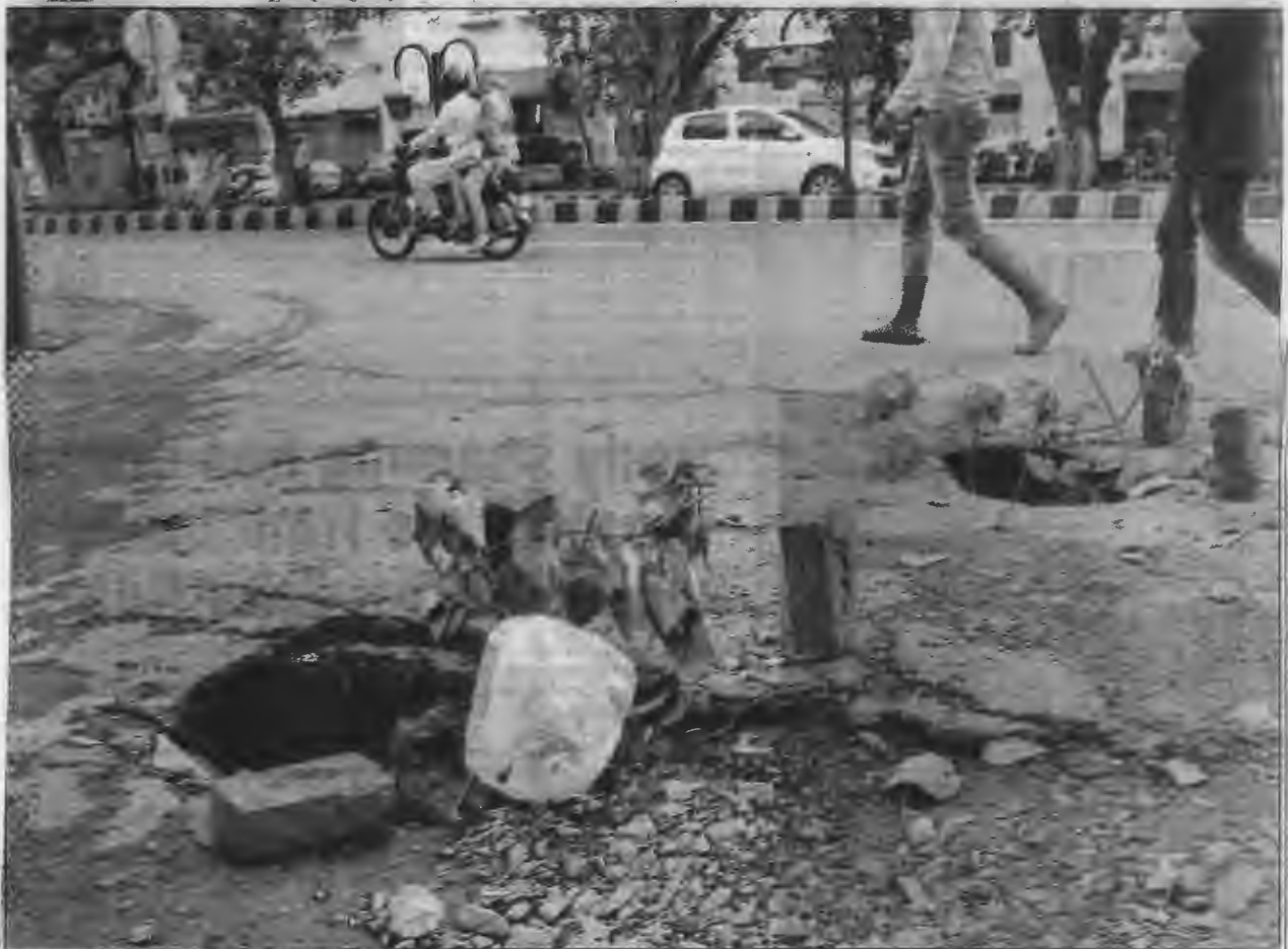
Two potholes appear along The Mall. Photo by Mansoor Ahmed
