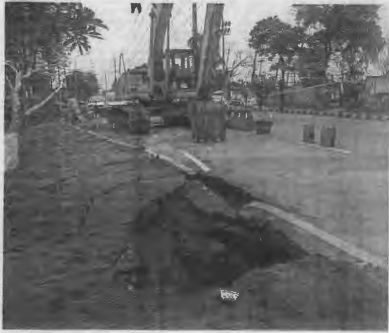
REPAIR work under way on a sinkhole which appeared on Johar Town main boulevard after rain on Sunday. — White Star
