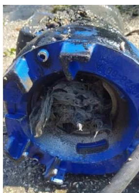
Pump Clogged by Wet Wipe
