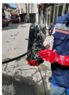
A piece of concrete dumped into a manhole
