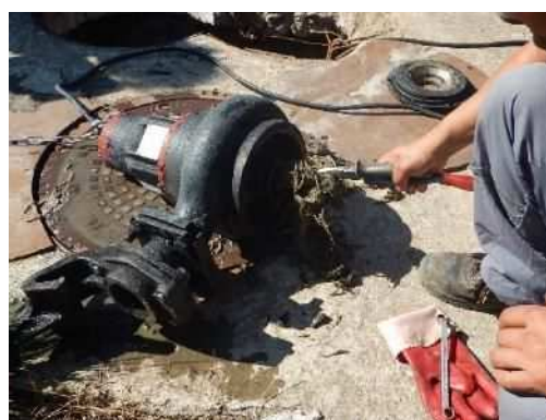
Removing wet wipes
