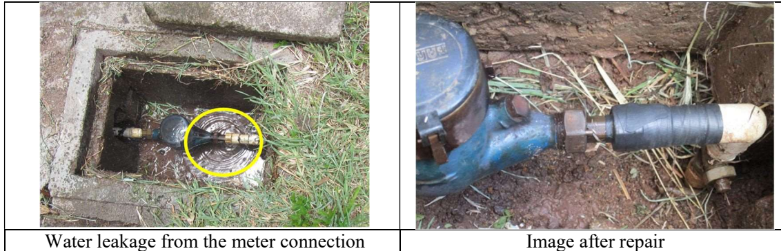
Figure 5-5-9 Leak and Repair Images
