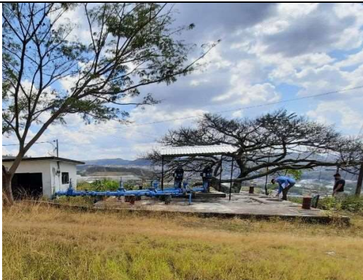
5. Pumping station No.25 Los Pinos
