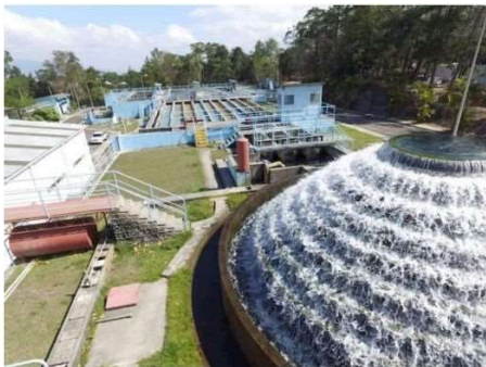
Photo 7 El Picacho Water Treatment Plant
