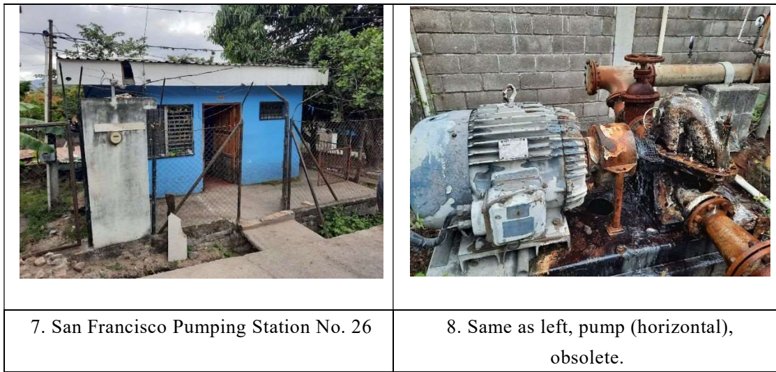
Figure 3-3-49 Status of Pumping Stations
