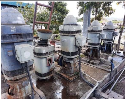
3. Pump at Nueva Suyapa pumping station No.8.
