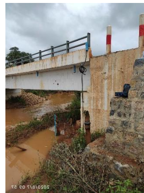
Water Level Gauge at the Bridge over Kalaw
