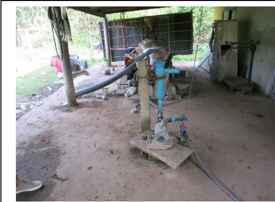
Photo-7 : A motor pump is installed in the riser pipe of the original hand pump.
