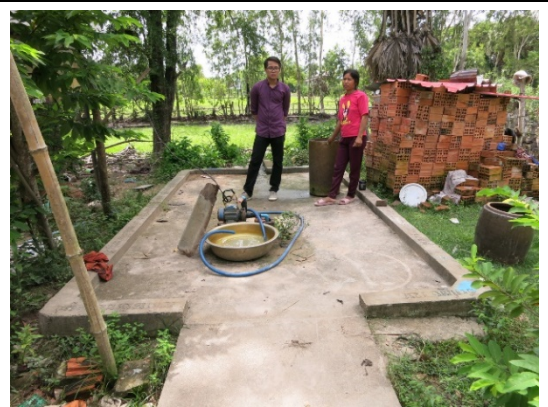
Photo-8 : A motor pump is installed in a hand pump well constructed by UNICEF.
