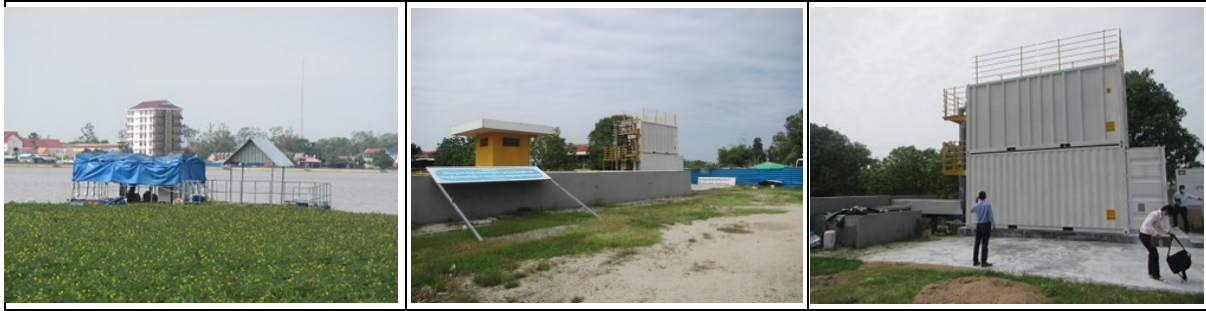
Note: Left: Intake Facility / Center & Right: Membrane Filter Source: Survey Team
