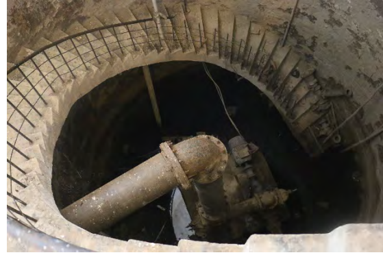
UNDERGROUND PUMP ROOM
