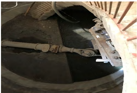
SUMBERSIBLE PUMP ROOM-2
