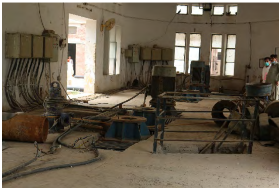
VERTICAL PUMP ROOM
