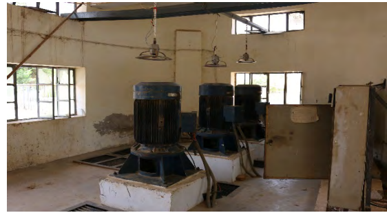
No.1 Pump Motor Room
