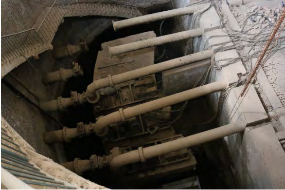
UNDERGROUND PUMP ROOM
