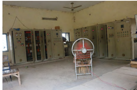
ELECTRIC CONTROL PANEL
