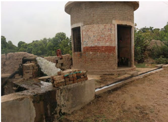
Pump discharge channel to farmland & Accompanying room
