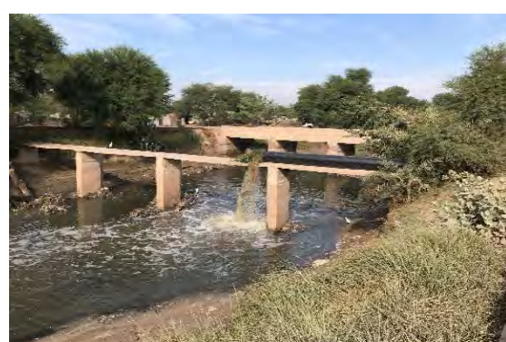
Discharge to Canal
