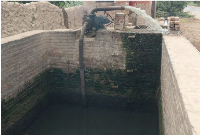
Pump and Pump Pit
