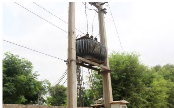
POLE – MOUNTED TRANSFORMER
