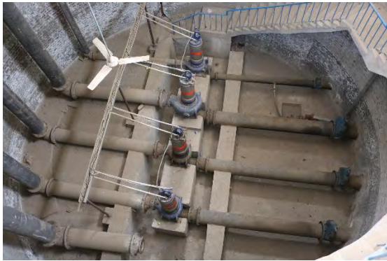
UNDERGROUND PUMP ROOM
