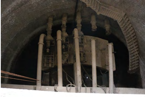
UNDERGROUND PUMP ROOM
