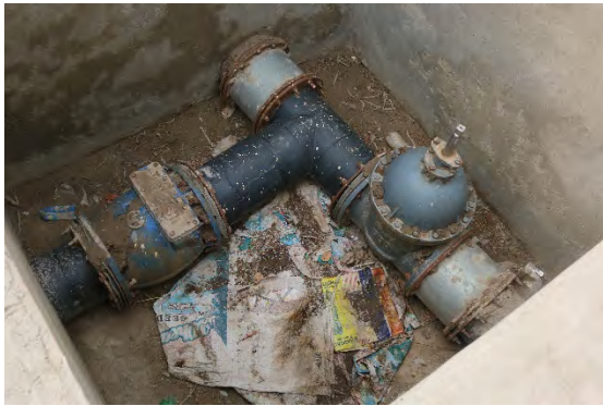
BRANCHED DISCHARGE PIPE
