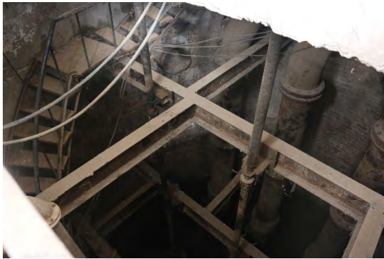
INTERMEDIATE SHAFT OF VERTICAL PUMP
