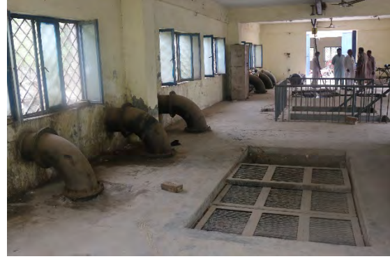
PUMP ROOM 1 F
