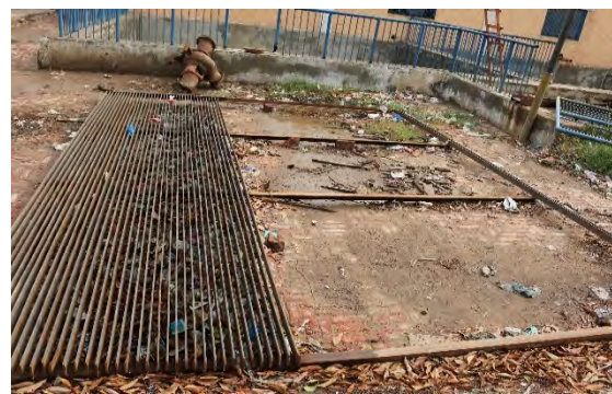
BROKEN RAKE SCREEN, WAITING FOR REPAIRS
