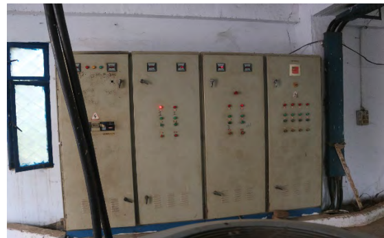
ELECTRIC CONTROL PANEL
