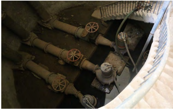
SUMBERSIBLE PUMP ROOM-1
