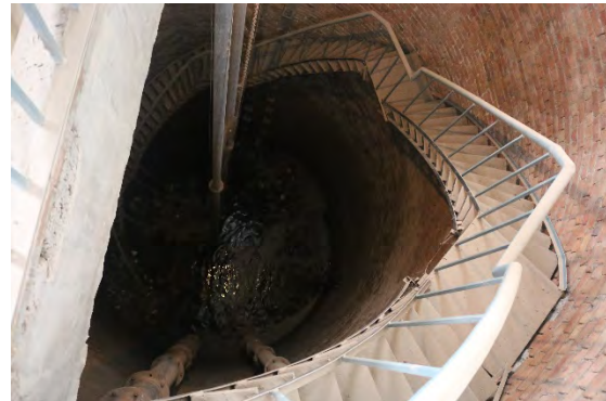
SUMBERSIBLE PUMP ROOM
