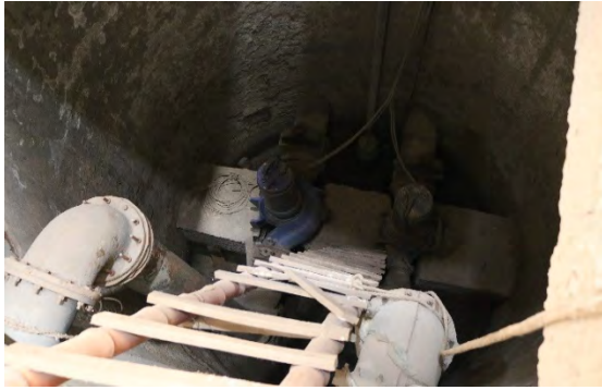
Underground pump room (SC)
