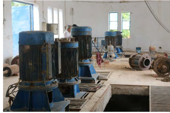
VERTICAL PUMP MOTOR ROOM
