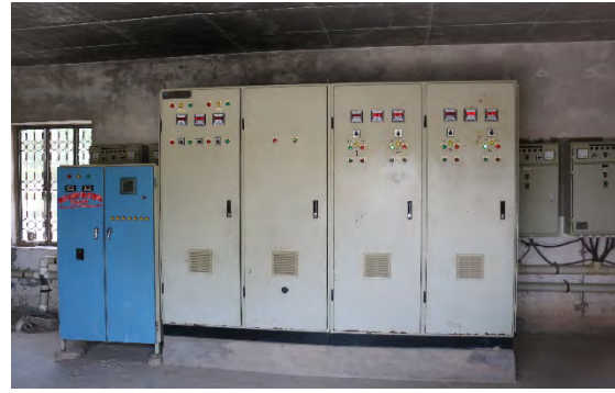
Electrical Room panel
