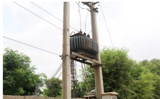
POLE – MOUNTED TRANSFORMER
