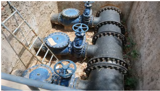
No.2 Pump discharge valve
