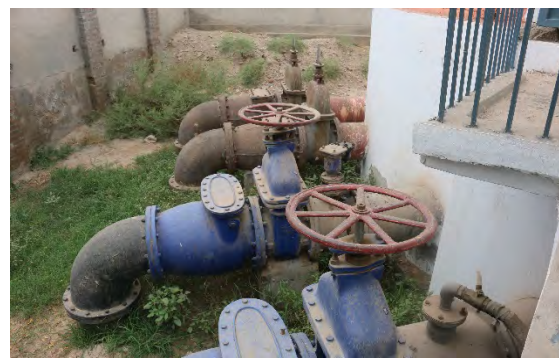
PUMP DISCHARGE VALVE
