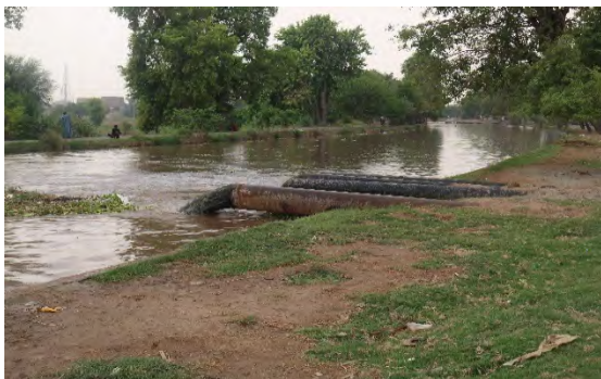
OUTFALL TO CANAL
