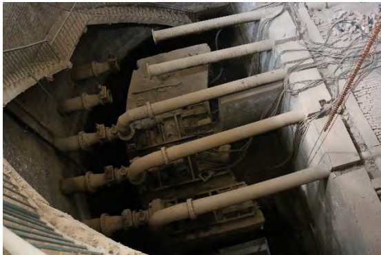
UNDERGROUND PUMP ROOM
