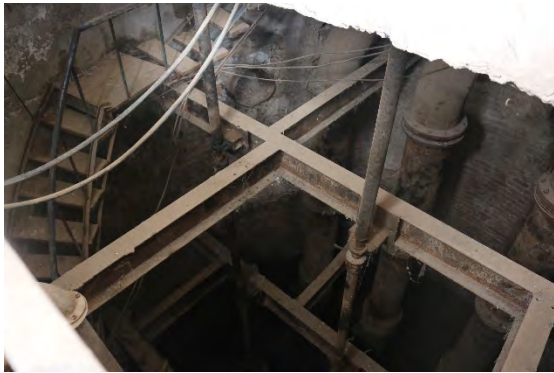
INTERMEDIATE SHAFT OF VERTICAL PUMP
