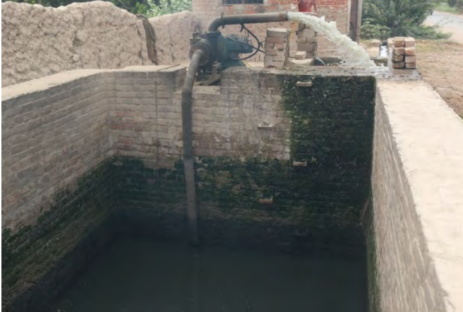
Pump and Pump Pit
