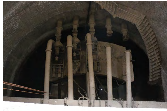
UNDERGROUND PUMP ROOM
