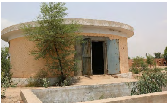
Pump Room 2 (New) submersible pump (SC)
