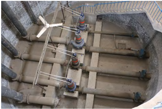
UNDERGROUND PUMP ROOM
