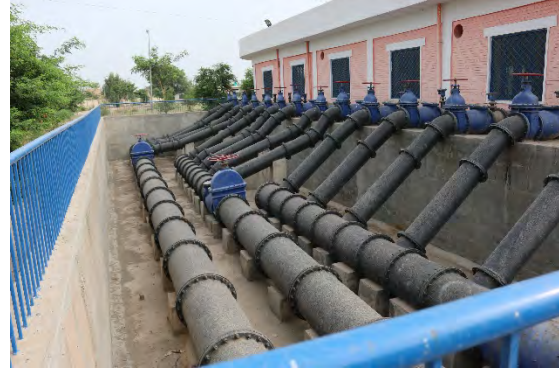
PUMP DISCHARGE PIPES
