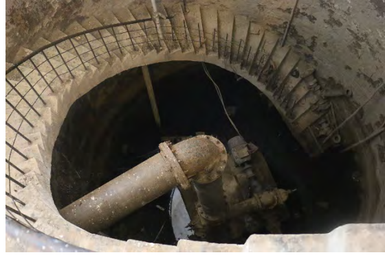
UNDERGROUND PUMP ROOM
