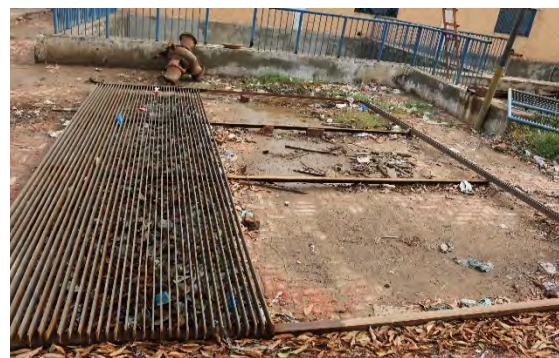
BROKEN RAKE SCREEN, WAITING FOR REPAIRS
