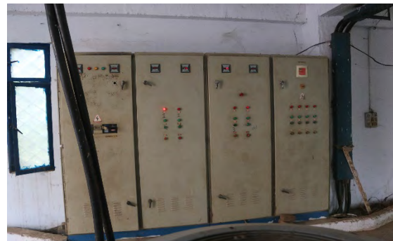
ELECTRIC CONTROL PANEL
