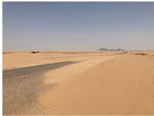
Section where pavement is covered with sand on Atbara-Haya Road
