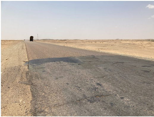
Road surface condition of Atbara-Haya road (Back side of road is constructed by China Front side of road is constructed by India)
