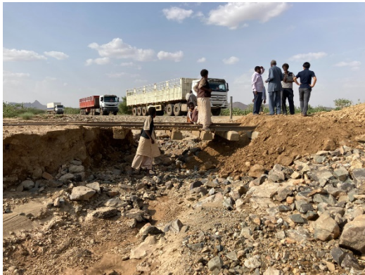
Flood washed roadbed and ballast of Sudan Railways Corporation's track
