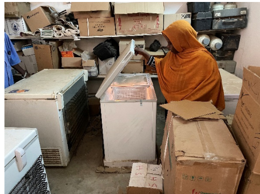
Vaccine Refrigerator at White Nile State susceptible to power outages, need solar panels installed
