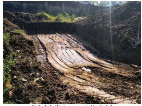
Photo-7: Wet Surface exposed at the trial pit
