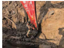
Fig. Damaged Pipe Found Being Repaired at Trial Pit Location
