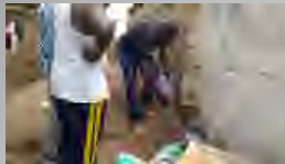
After disconnected with plug as usual, the customer illegally removed meters(?). POC=202212054
