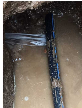
Photo 2 A water leak
