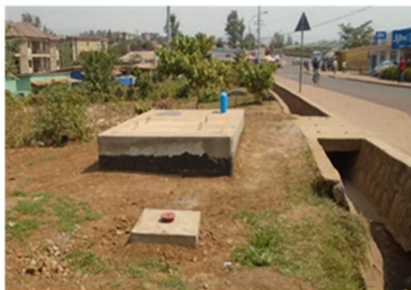
Water meter chamber and valve chamber
