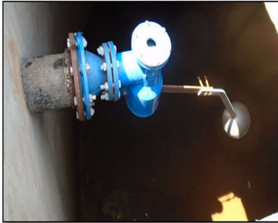
Figure 3 . floater valve installed in the reservoir
