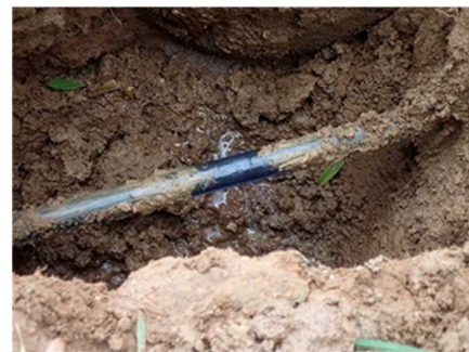
Minor water leak from a tertiary pipe
