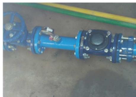
Inside of water meter chamber
