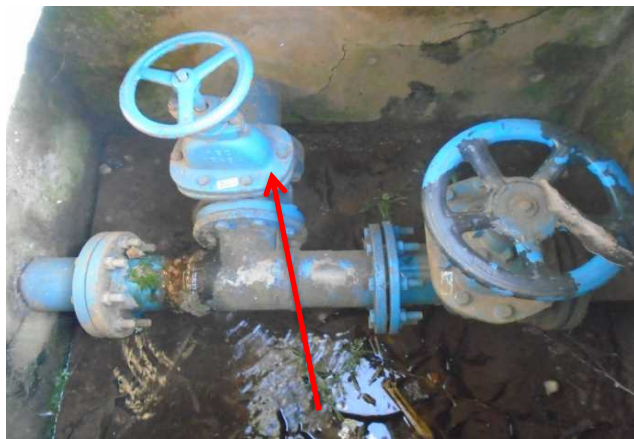
Inlet Pipe with Valve
