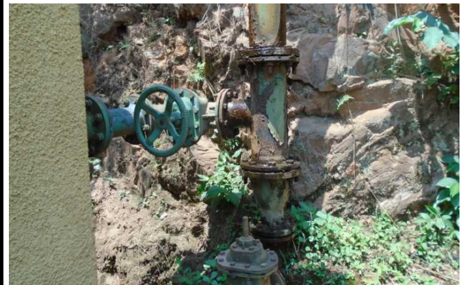
Outlet Pipe with Valve
