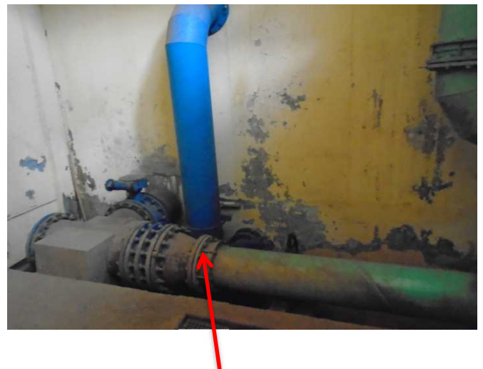
Outlet Pipe with Valve
