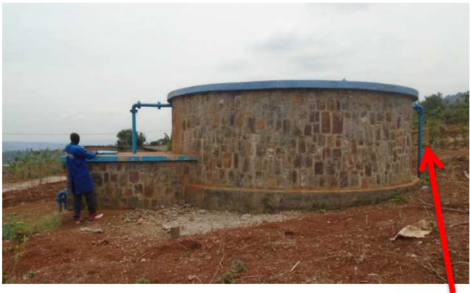
Inlet Pipe without Valve
