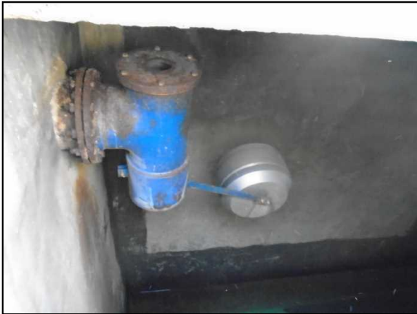
Defective floater valve
