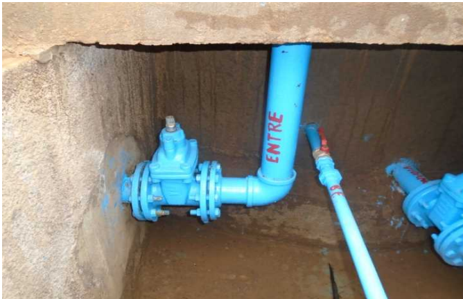
Inlet Pipe with Valve
