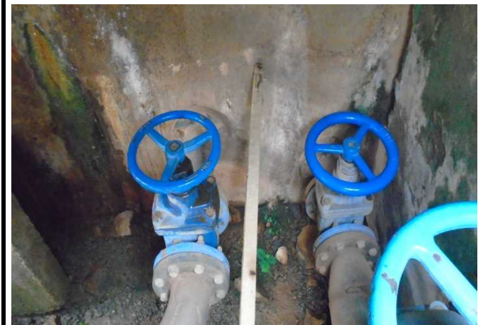
Outlet Pipe with Valve
