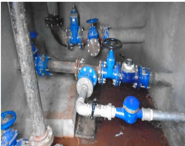
Inlet Pipe with Valve
