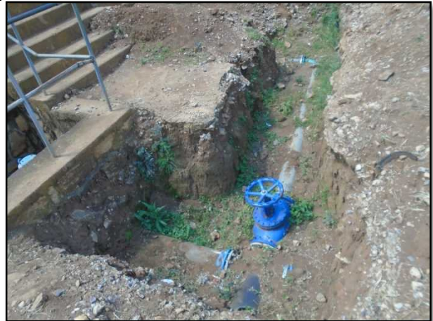
Backfilling and construction of a protection manhole is needed
