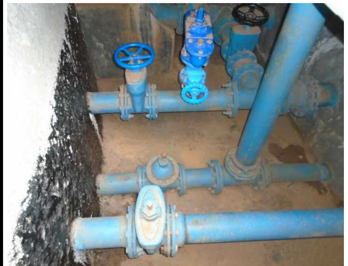
Outlet Pipe with Valve
