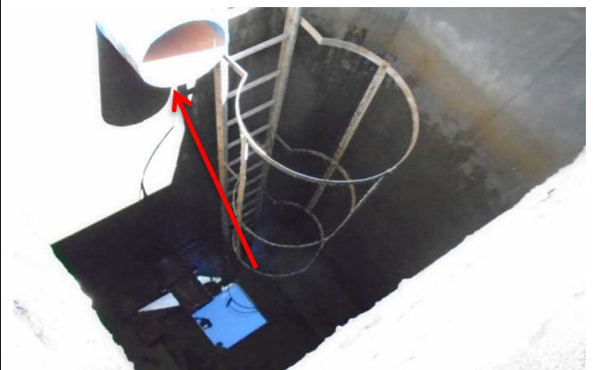
Outlet Pipe with Valve
