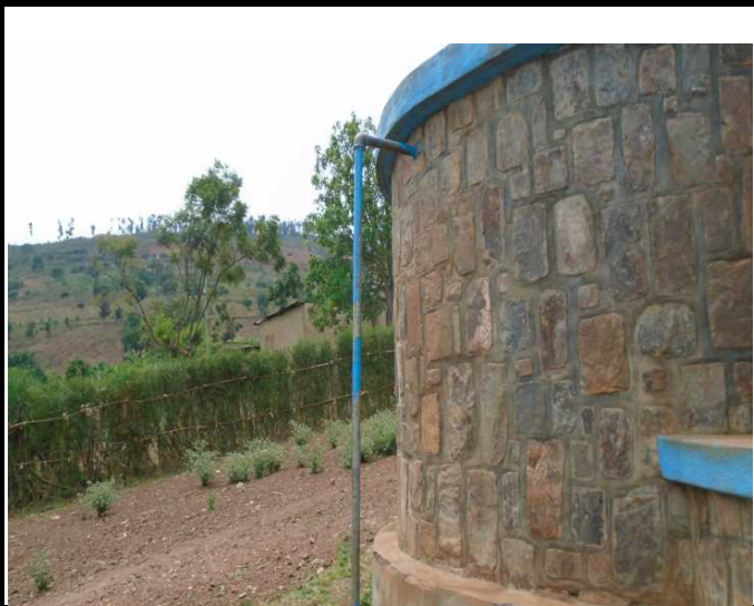
Inlet Pipe without Valve
