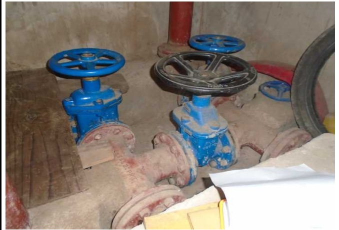
Outlet Pipe with Valve
