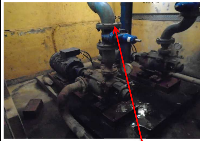
Outlet Pipe with Valve
