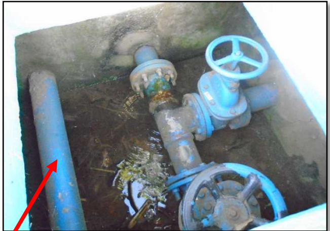
Inlet pipe without drainage
