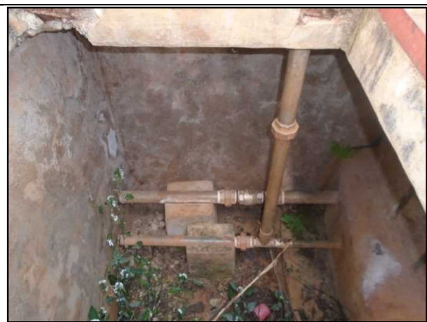
Manhole need a cover
