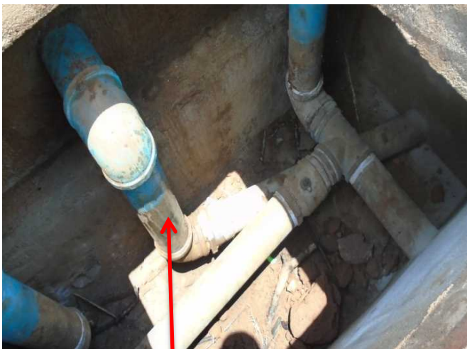
Inlet Pipe with Valve
