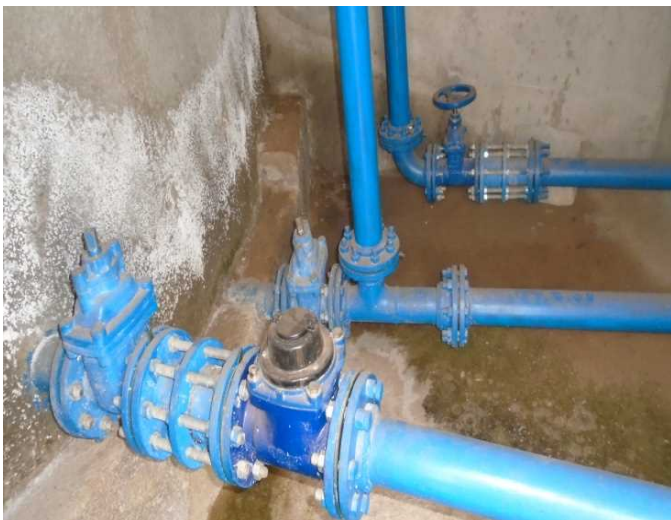
Inlet Pipe with Valve
