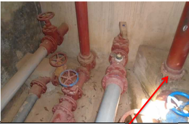
Inlet Pipe with Valve
