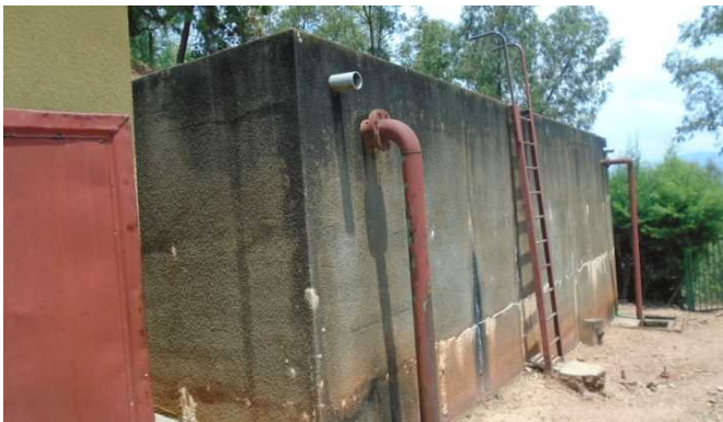
Inlet Pipe with Valve
