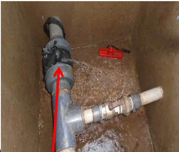
Inlet Pipe with Valve
