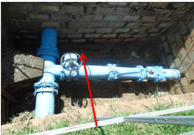
Inlet Pipe with Valve
