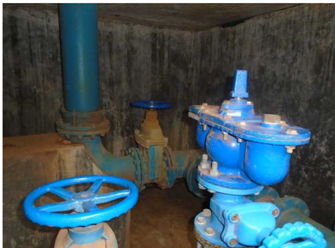
Inlet Pipe with Valve
