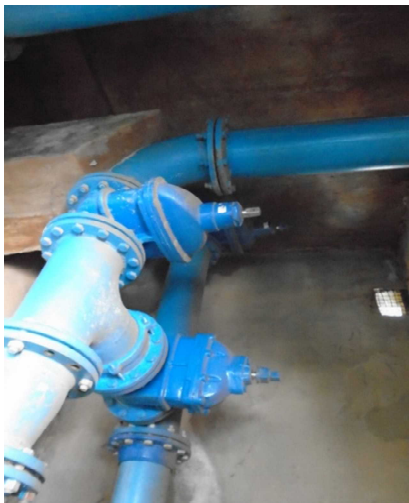
Inlet Pipe with Valve
