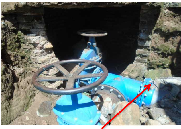
Inlet Pipe with Valve
