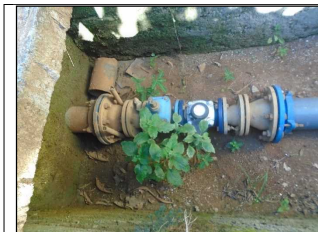
Inlet Manhole Needed
