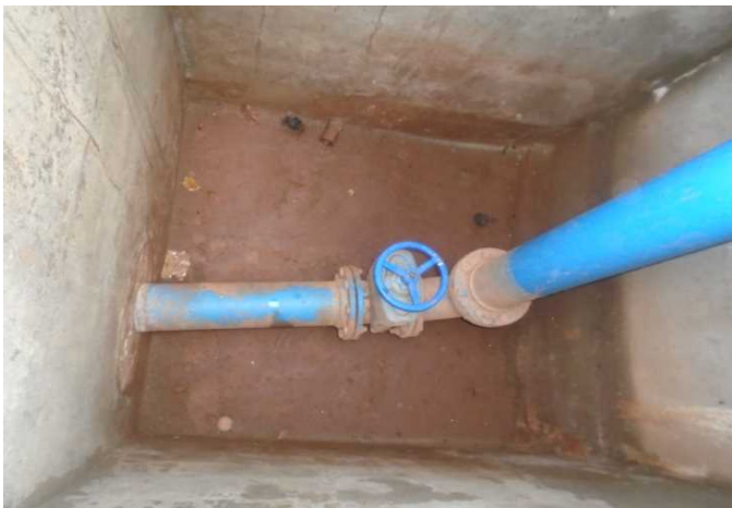
Inlet Pipe with Valve
