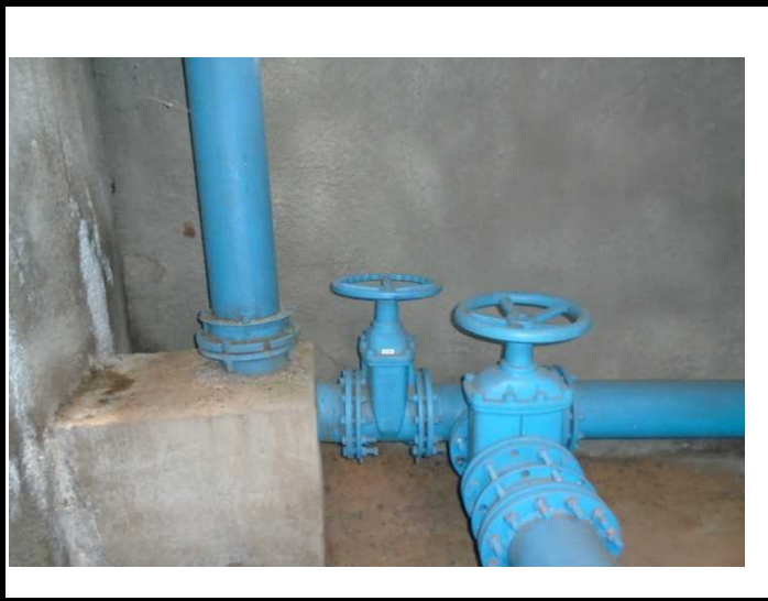
Inlet Pipe with Valve
