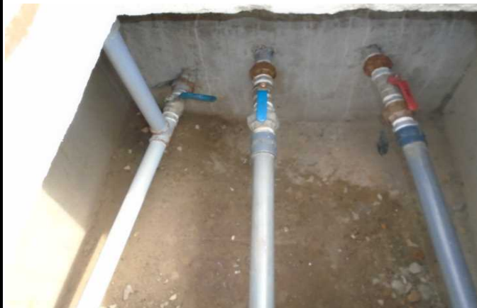
Inlet Pipe with Valve
