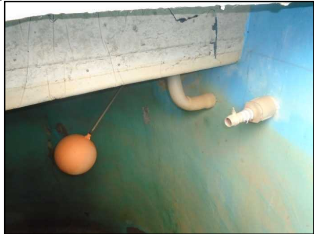
Installed floater not working
