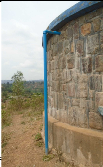
Inlet Pipe without Valve
