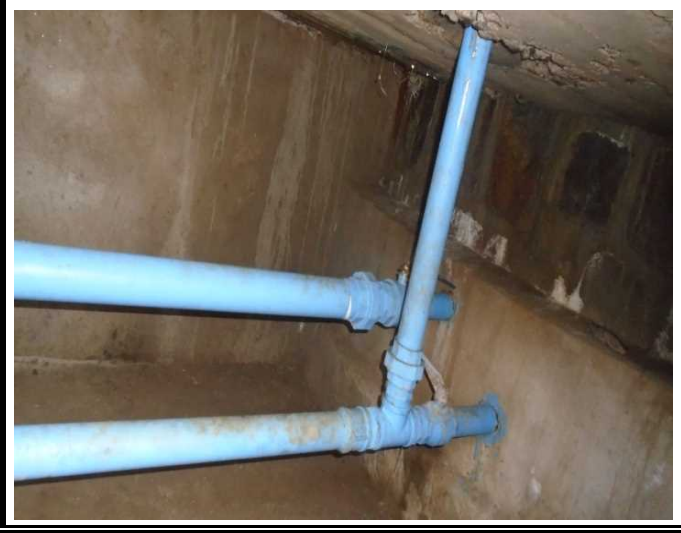
Outlet Pipe with Valve
