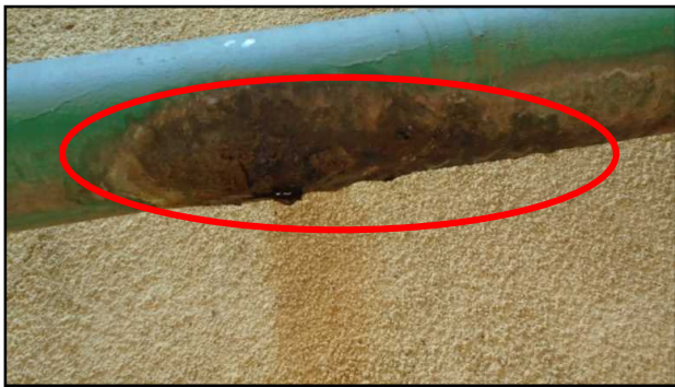
Leaking pipe to be replaced
