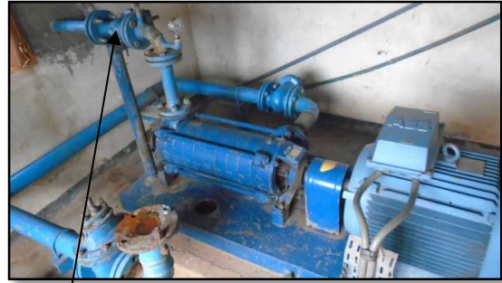
Check valve to replace
