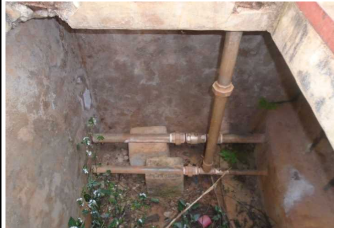
Outlet Pipe with Valve
