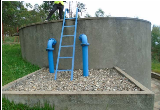
Inlet Pipe with Valve
