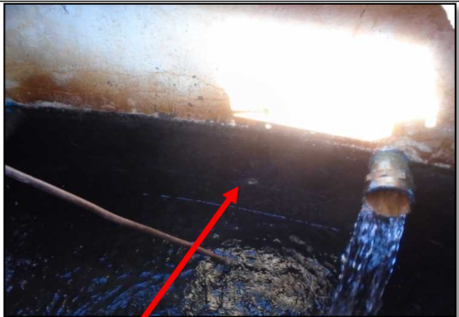
Crack on the wall (entrance of flood water)
