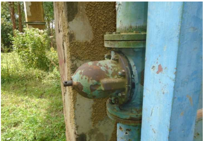
Inlet Pipe with Valve
