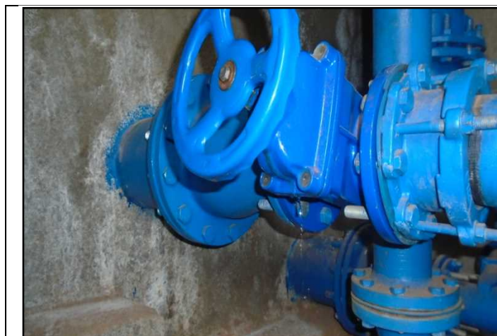
Leaking Outlet Valve
