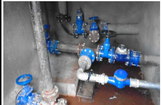
Outlet Pipe with Valve
