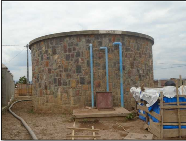
Cracks on the wall leaking.
