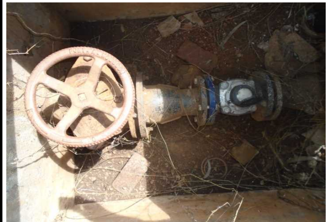
Outlet Pipe with Valve
