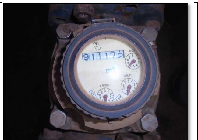
Meter on Ntora pipe need checking
