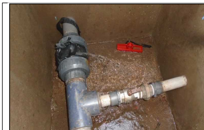
Leaking Inlet PVC Valve
