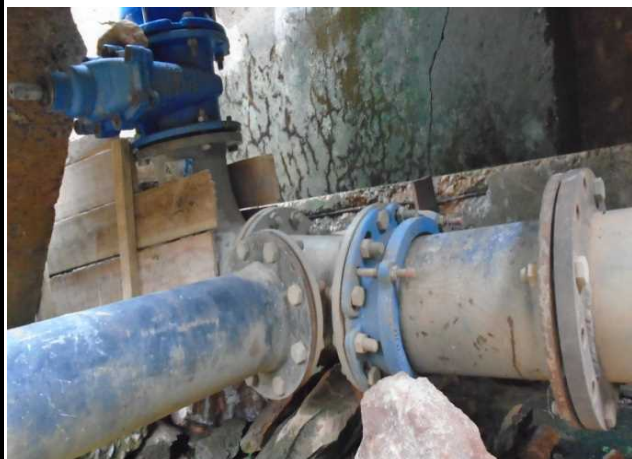
Inlet Pipe with Valve
