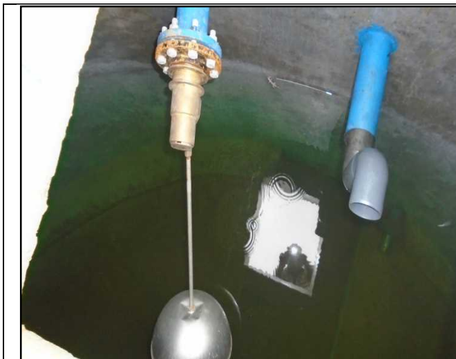
Floater Valve which doesn't fully close.
