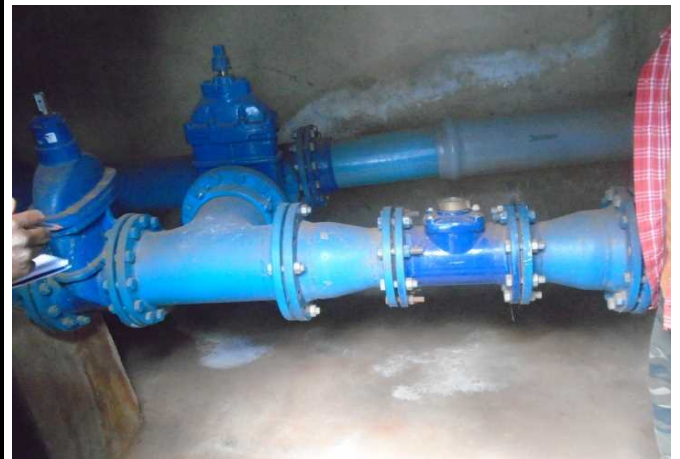
Outlet Pipe with Valve
