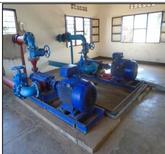
Pumps also connected to the old support Reservoir
