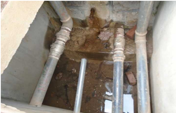
Inlet Pipe with Valve
