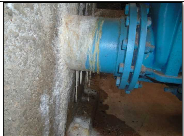
Leak at the bottom of drain pipe need fixing
