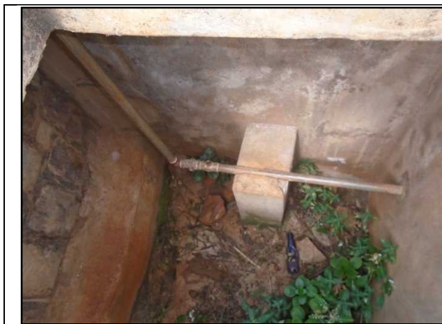
Inlet valve need to be replaced
