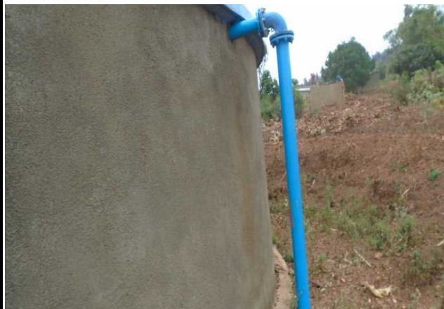
Inlet Pipe without
