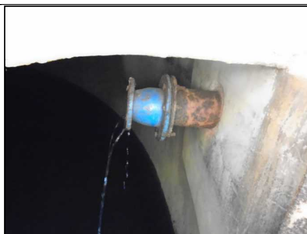
No floater valve installed
