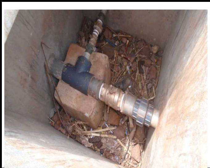
Outlet Pipe with Valve
