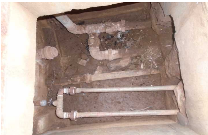
Inlet Pipe with Valve
