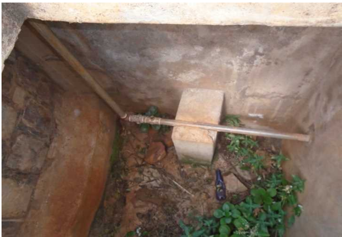
Inlet Pipe with Valve
