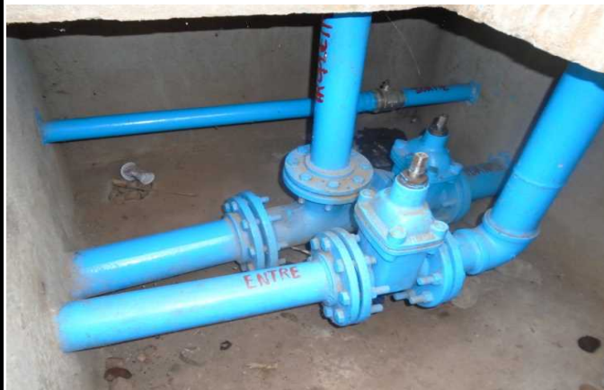
Inlet Pipe with Valve
