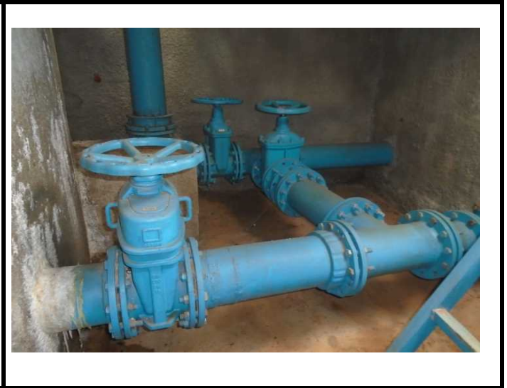
Outlet Pipe with Valve
