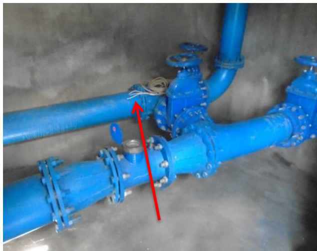
Inlet Pipe with Valve
