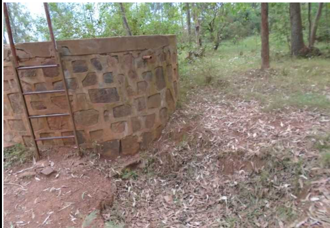
No Inlet Pipe
