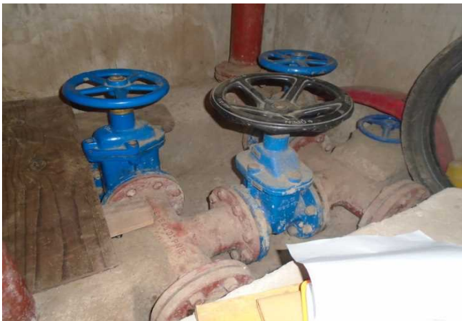
Inlet Pipe with Valve
