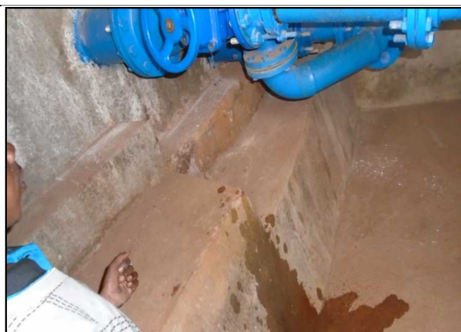
Valve leaks when opened
