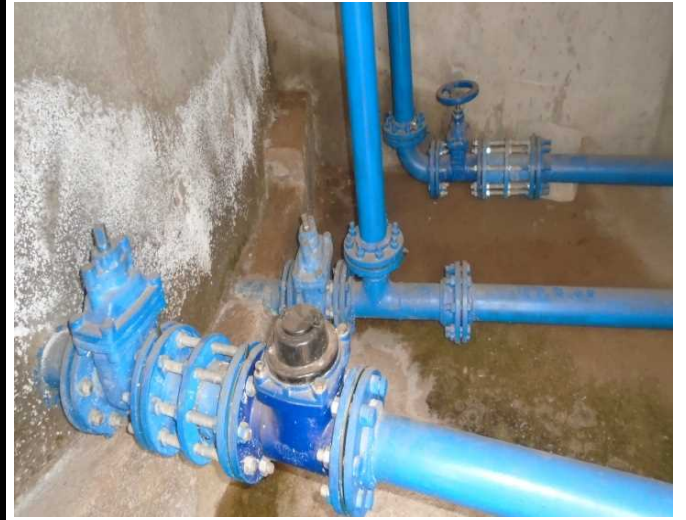
Outlet Pipe with Valve
