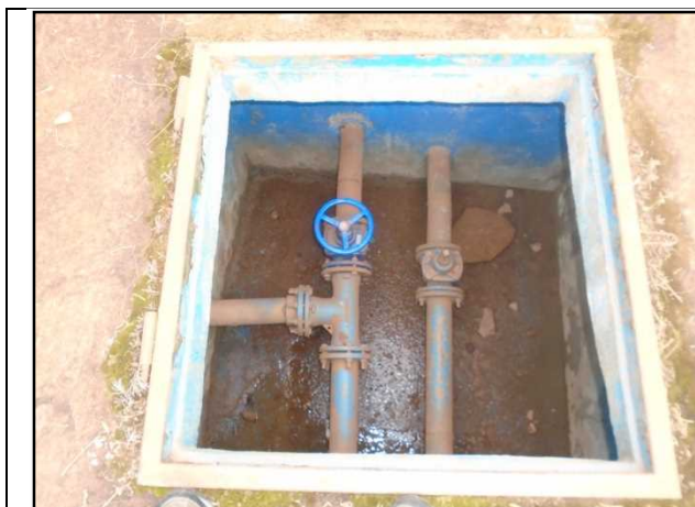
Leaking bypass valve
