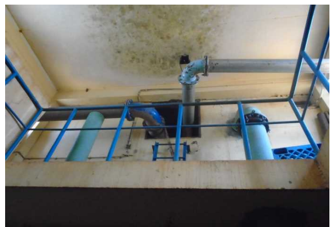
No Floater Valves installed for the whole 3 pipes
