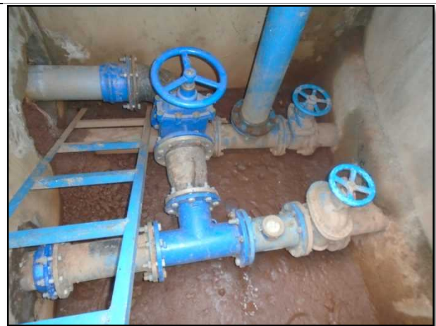
Manhole drainage system
