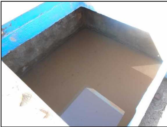
Reservoir drainage Valve manhole full of water
