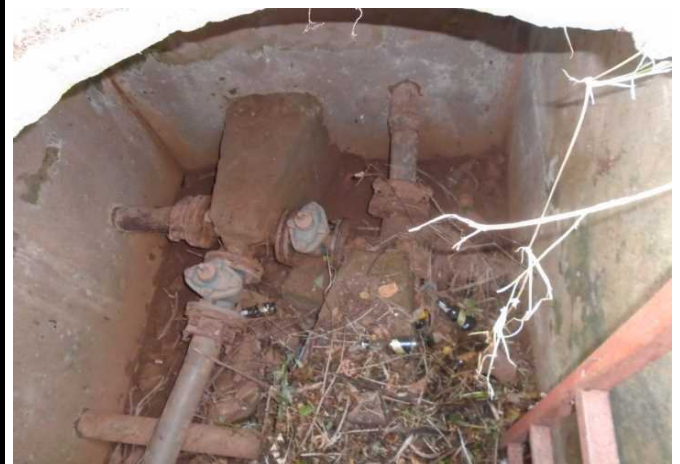
Outlet Pipe with Valve
