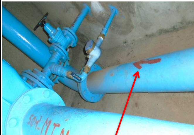
Inlet Pipe without Valve
