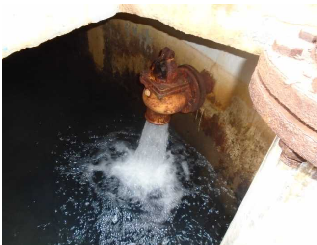
Inlet Pipe with Valve
