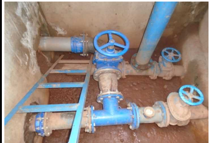
Outlet Pipe with Valve
