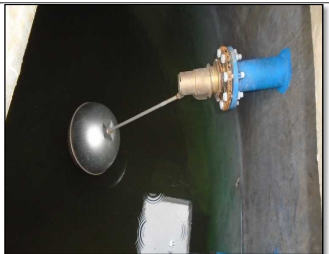
Floater Valve which doesn't fully close.
