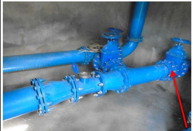
Outlet Pipe with Valve
