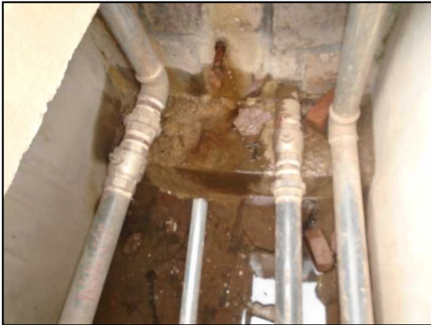
Outlet towards Public Water Tap Leaking
