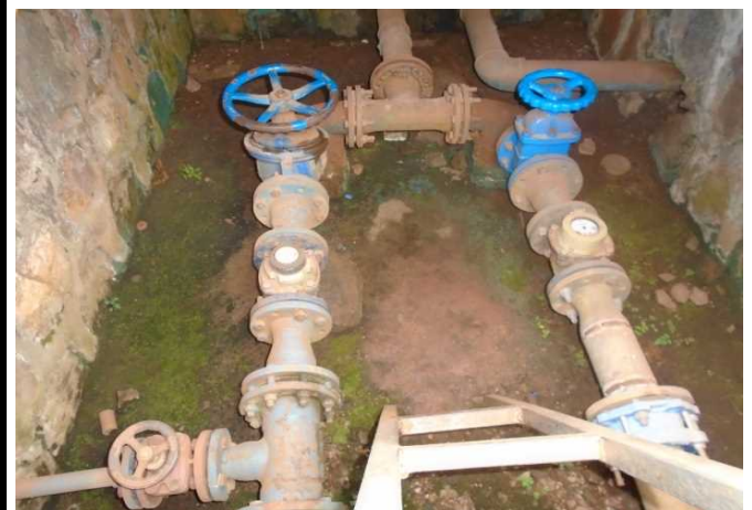
Outlet Pipe with Valve
