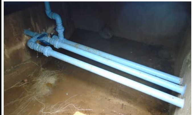
Outlet Pipe with Valve
