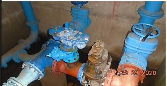
Outlet Pipe with Valve
