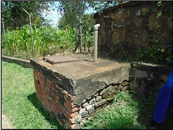
Inlet connection and valve
