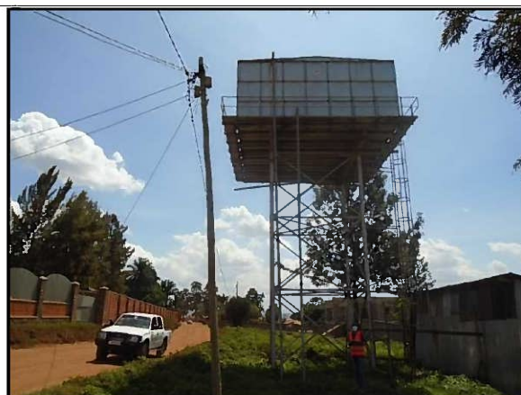
Overflow pipe and drain pipe needed
