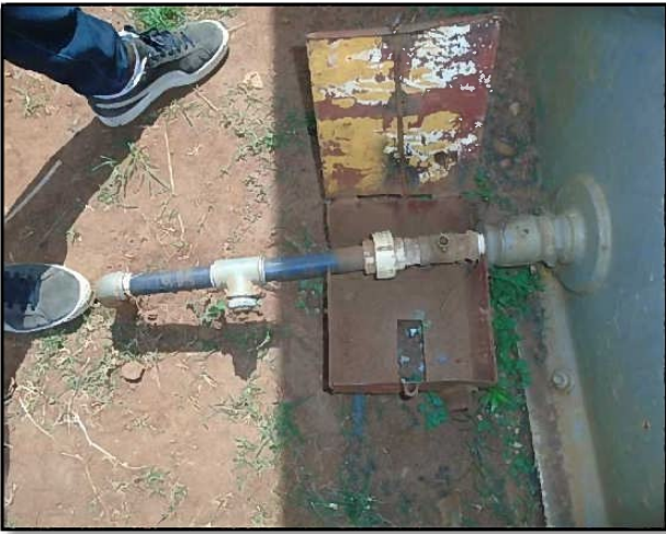
Outlet valve need to be replaced.
