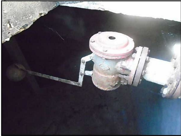
Defective floater valve
