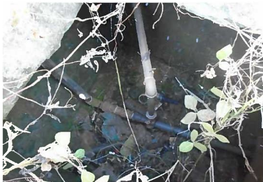
Inlet Pipe with Valve
