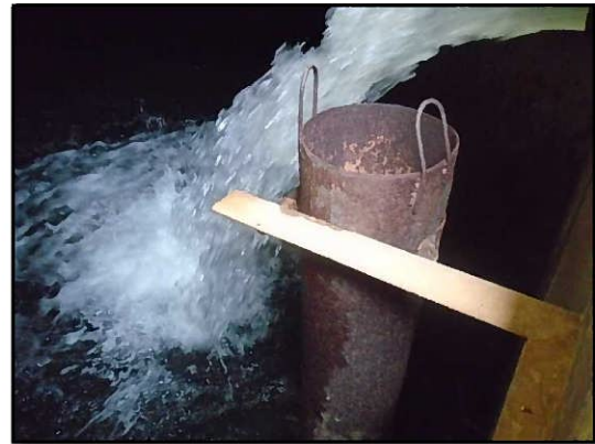
Overflow Pipe defective (if possible replacement is recommended)
