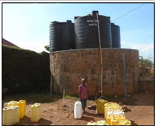
The whole reservoir needs general rehabilitation.
