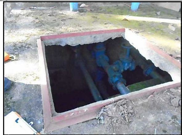
New covers needed for manhole and Reservoir
