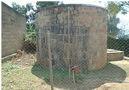
Inlet Pipe with Valve
