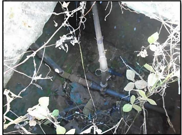
Inlet and outlet manholes need covers
