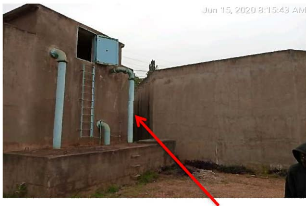
Inlet Pipe with Valve
