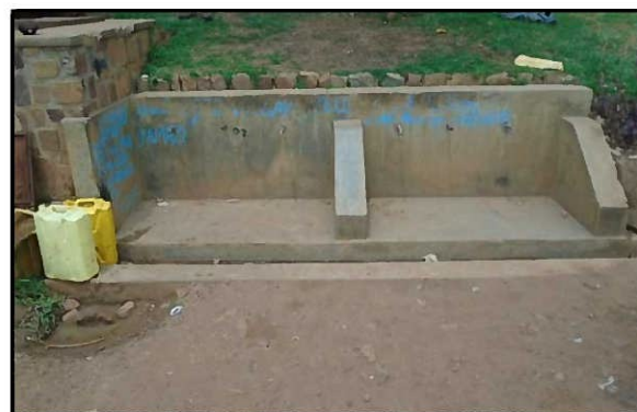
Water tap Valves needed.
