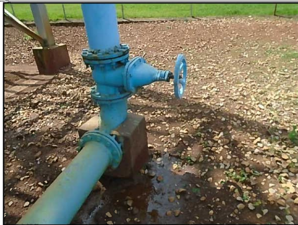
Defective inlet valve
