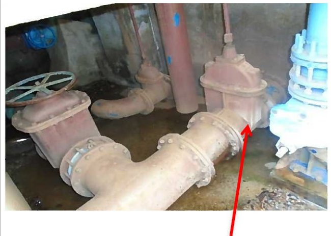
Outlet Pipe with Valve
