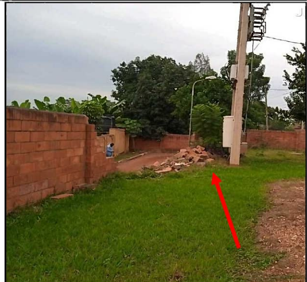
These fallen part of fence are being used by thieves and intruders
