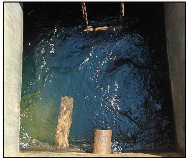
Floater valve needed + general maintenance of the tank
