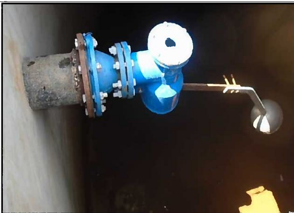
Installed floater valve not functional
