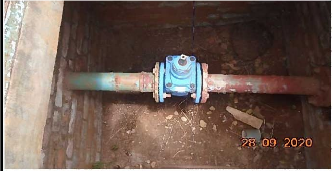
Outlet Pipe with Valve
