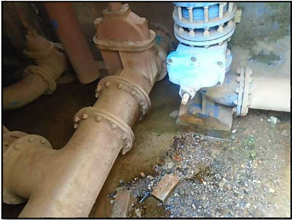
Defective Leaking vertical valve
