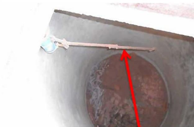
Float Valve Defective
