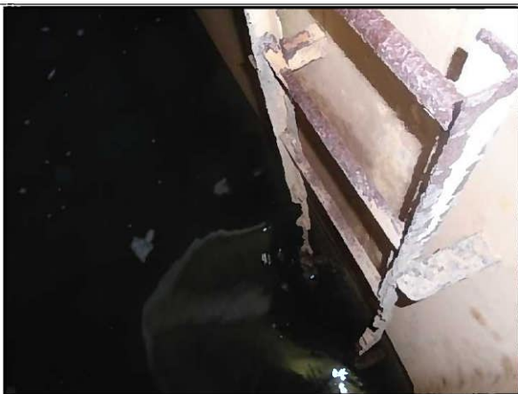
Stairs need replacement
