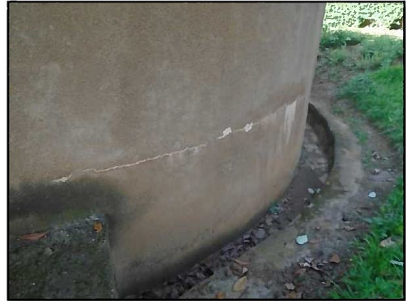
Rehabilitation needed to waterproof it as it was abandoned because it was leaking on walls and base
