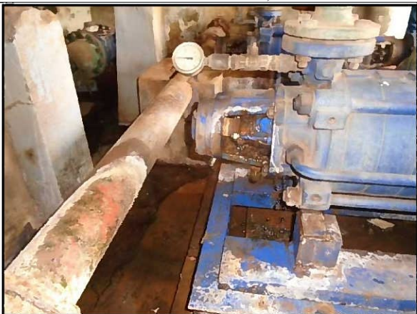
Pump with a Pressure Gauge which doesn't work
