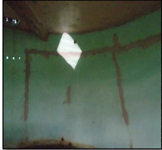
Cracks on the wall and need
