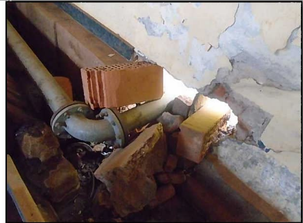
Pump House needs maintenance
