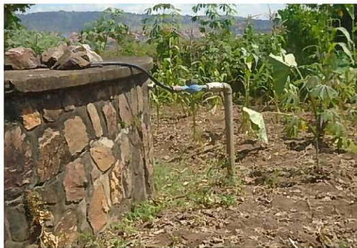
Inlet Pipe with Valve
