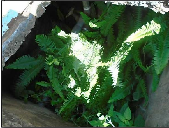
General maintenance works needed
