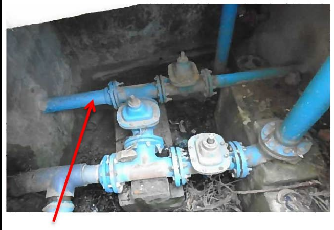
Outlet Pipe with Valve
