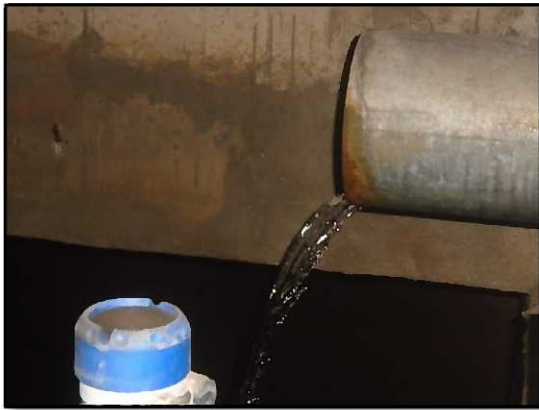
No Floater Valve installed
