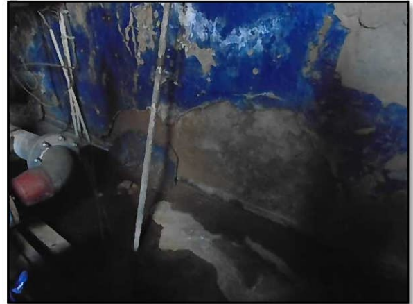
Rehabilitation needed for pump house
