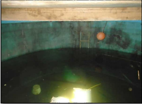
Floater Valve need Repairing or replacement
