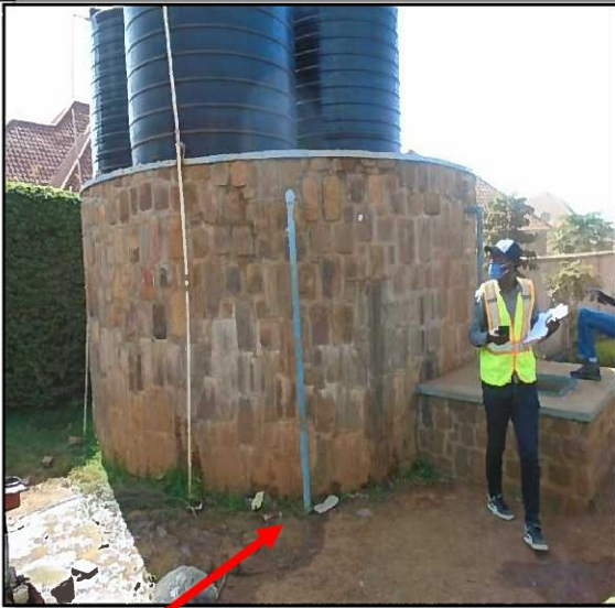
Inlet pipe needs a manhole and a valve.
