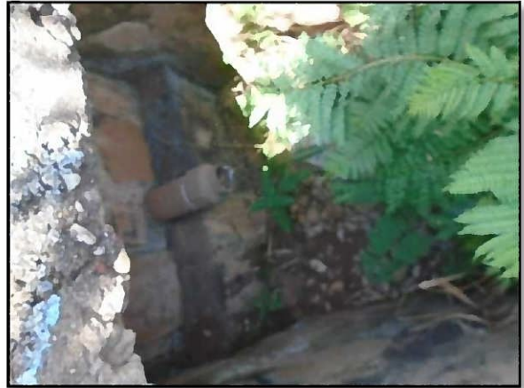
Recennection and outlet valve needed
