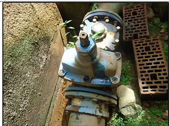
Inlet valve Res.2 need replacement
