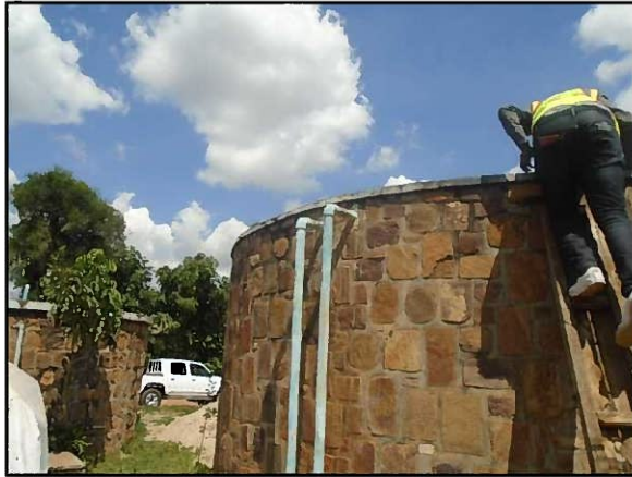
Floater valve needed for inlet pipe
