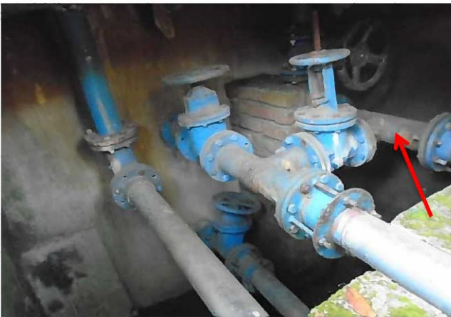
Inlet Pipe with Valve
