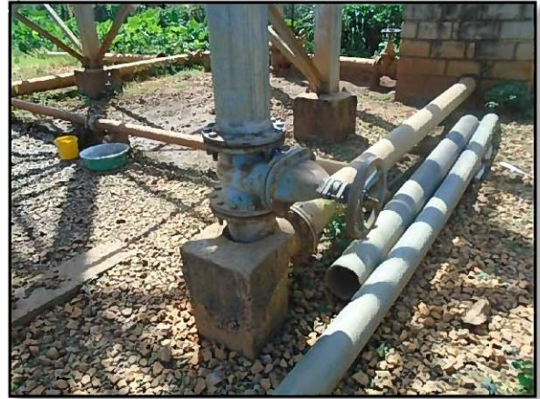
Valve support of thrust blocks (all) need rehabilitation.
