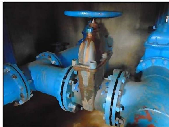
Bypass valve leaking
