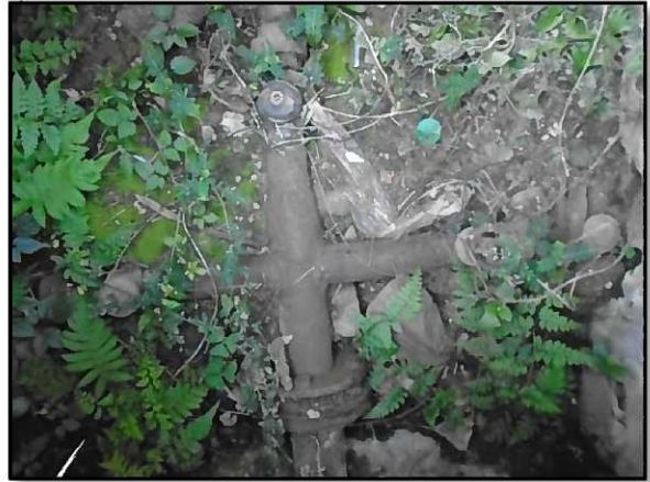
Outlet network need rehabilitation
