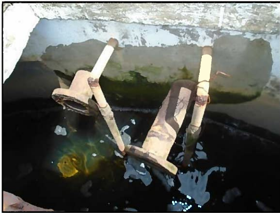
Inlet from Rwampara DN100 (no inlet valve or Floater valve)
