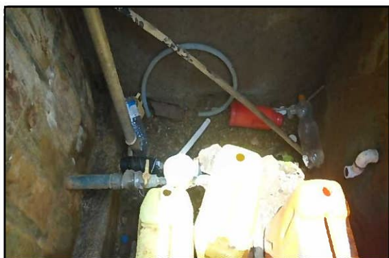
Outlet and drainage valves needed.
