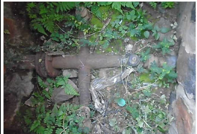
Outlet Pipe with Valve
