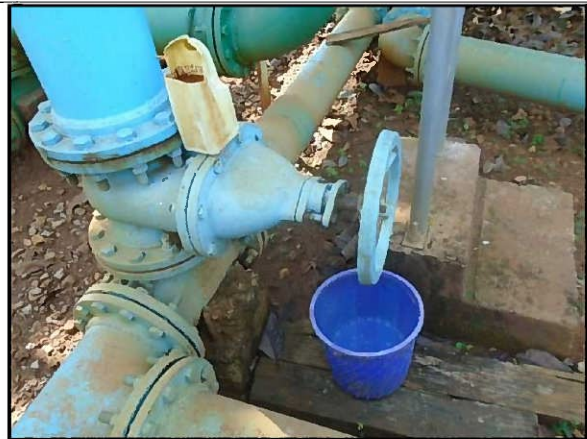
Defective Outlet valve
