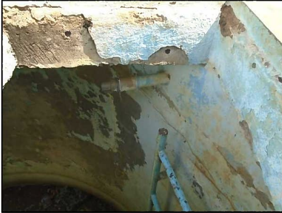
No floater valve installed
