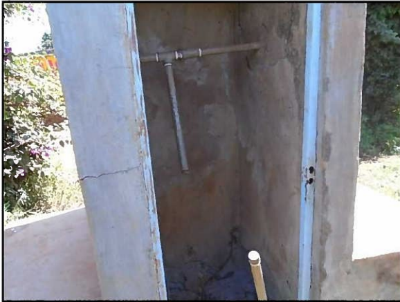
Water tap reconnection recommended
