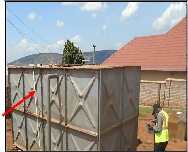
Inlet pipe need to be fixed and connected to the roof opening of the tank.
