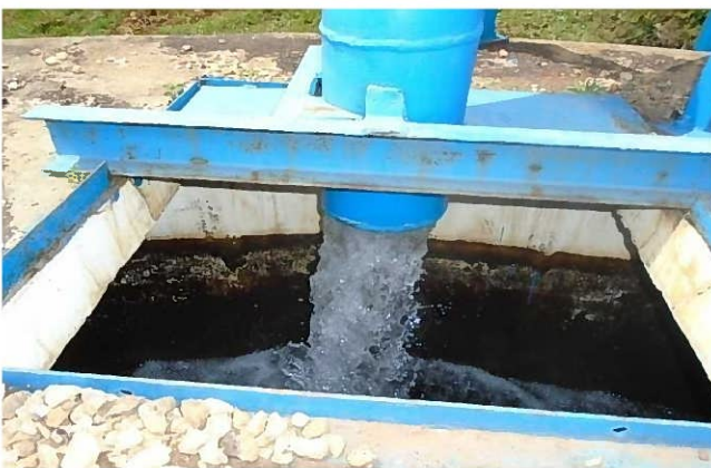
No Float Valve installed
