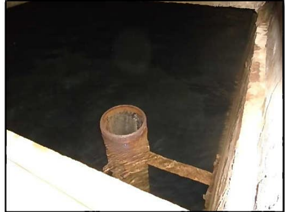
General accessories cleaning needed as soon as possible
