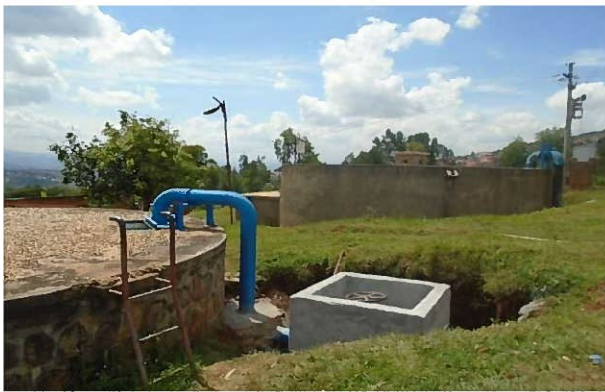
Inlet Pipe with Valve
