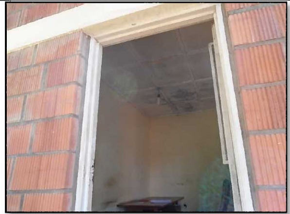
Operator house leaking
