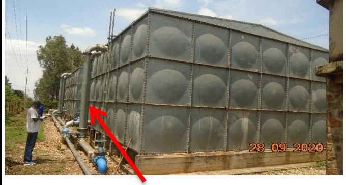
Inlet Pipe With Valve
