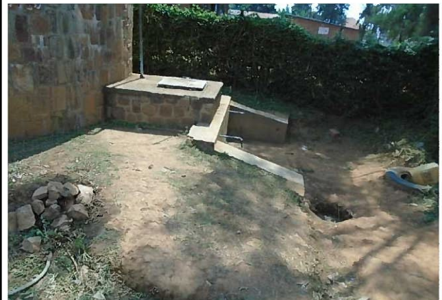
Outlet Pipe with Valve
