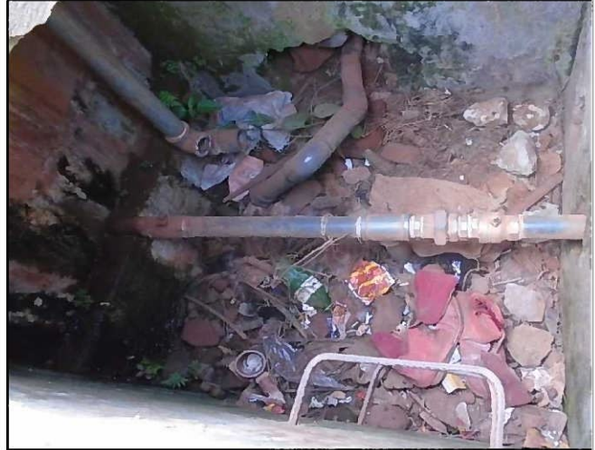
Outlet manhole need rehabilitation, cover and pipe reconnection
