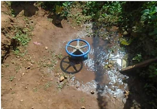
Inlet Pipe with Valve
