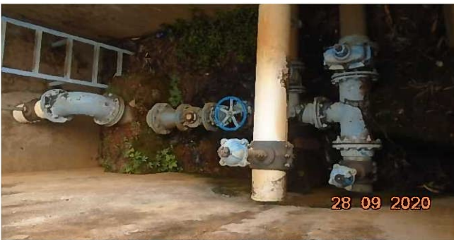
Inlet Pipe with Valve
