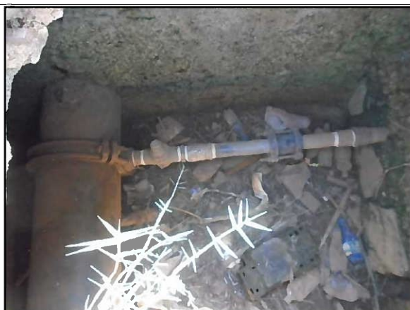
Installation of a Meter needed
