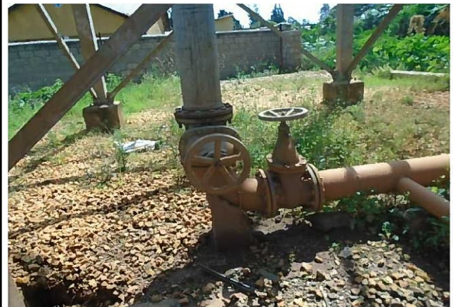
Outlet Pipe with Valve
