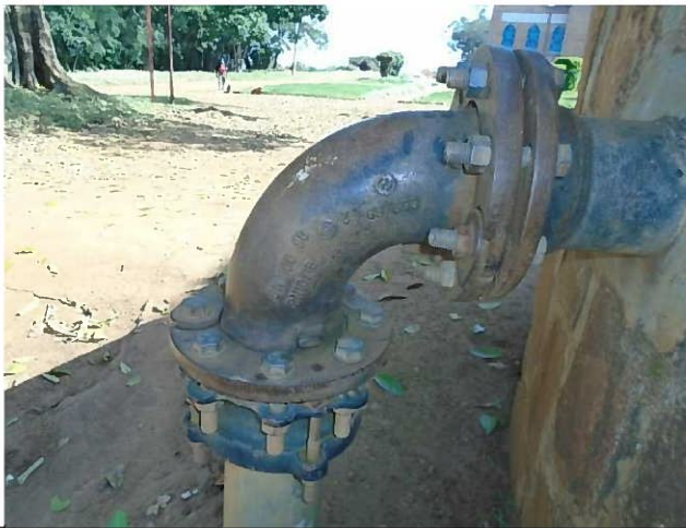
Inlet Pipe with Valve
