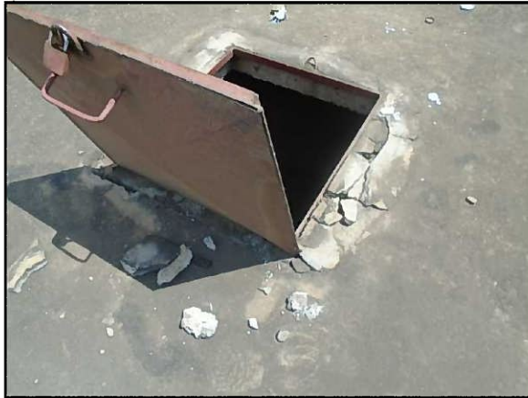
Cover protection maintenance needed
