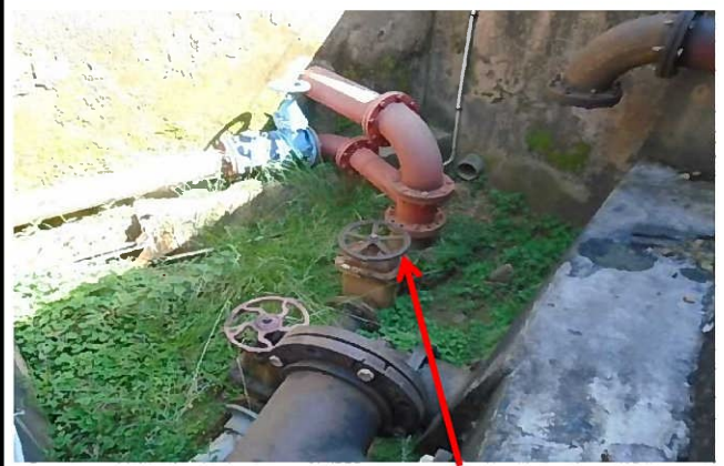
Outlet Pipe with Valve
