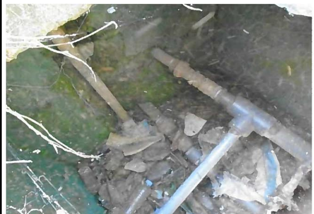
Outlet Pipe with Valve
