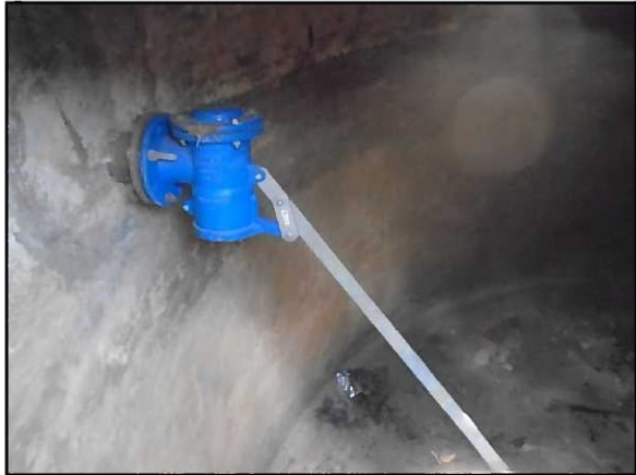
Defective floater valve
