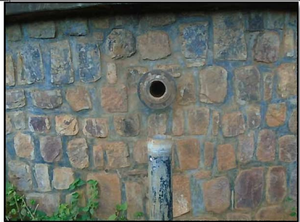
Reconnection will be needed
