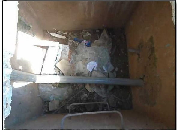
Reconnection and inlet valve needed
