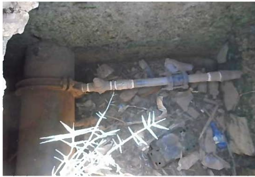
Inlet Pipe with Valve
