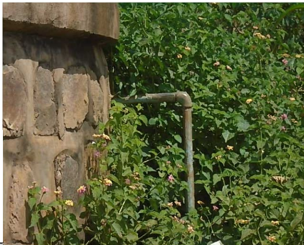
Inlet Pipe with Valve
