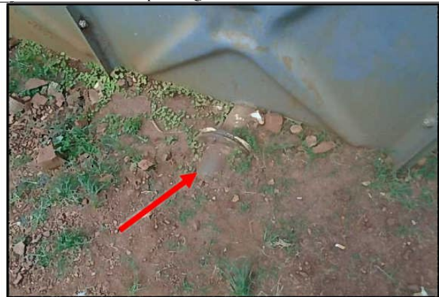
Drain pipe need a valve and a manhole
