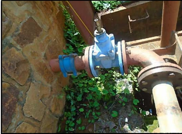
Inlet valve not operational
