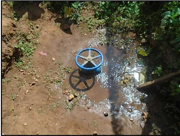
Inlet valve leaking
