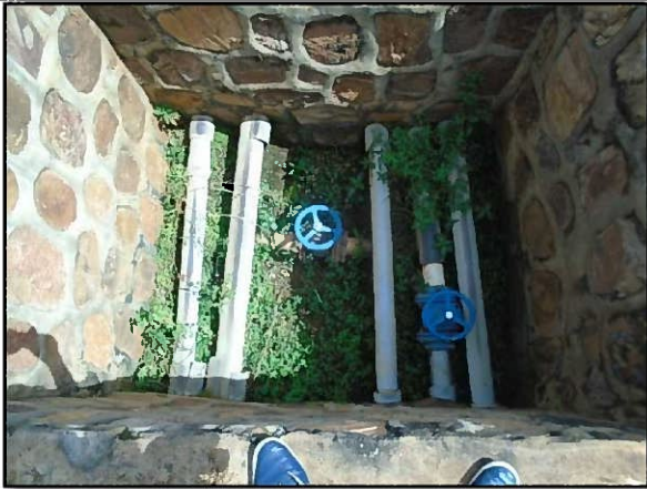
Drainage is need for 3 of the 5 inlet pipes
