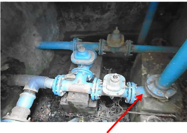
Inlet Pipe with Valve
