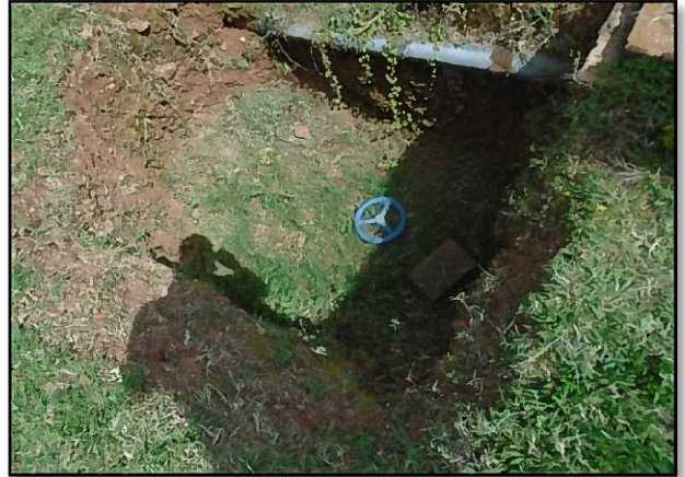
Collection Chamber drainage valve
