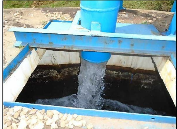
Inlet from Nzove Pipe DN300 (No floater)
