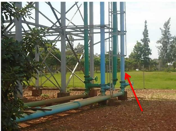
Inlet Pipe with Valve
