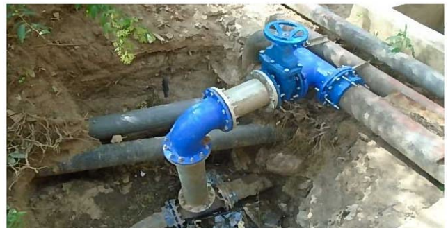
No Meter (Photo: Network modified and reservoir bypassed)
