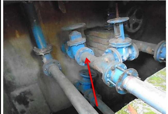
Outlet Pipe with Valve
