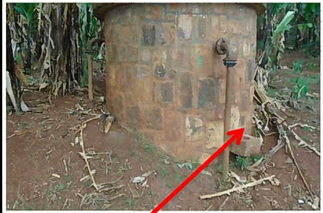
Outlet Pipe with Valve
