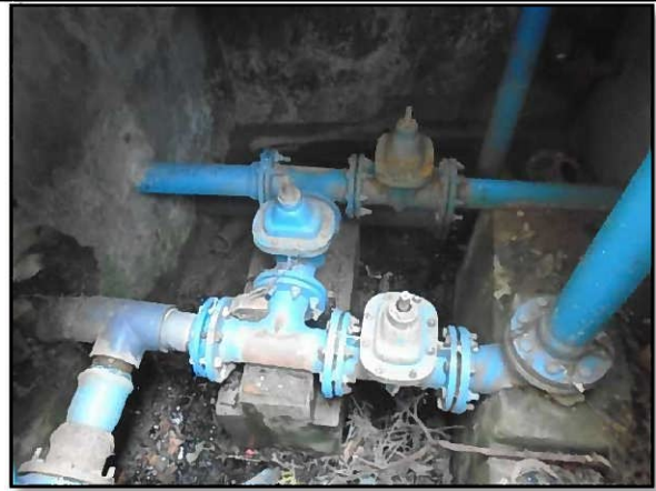
General cleaning works needed.
