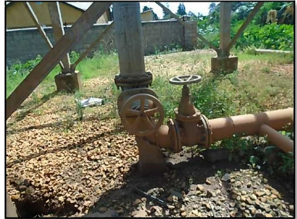
Outlet valve not operational
