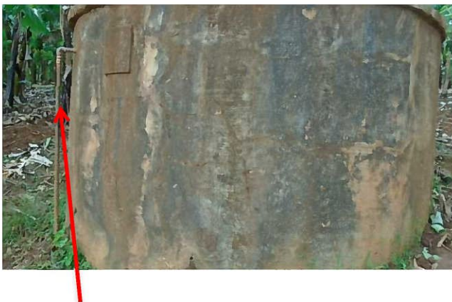
Inlet Pipe with Valve
