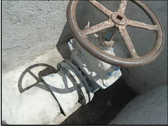
Inlet from Nzove Valve DN300 (Not working)
