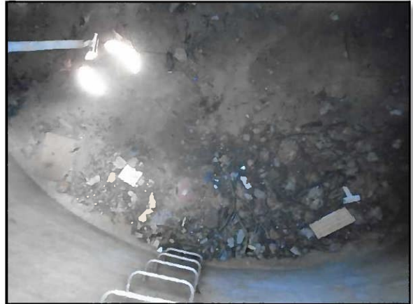
General rehabilitation is needed
