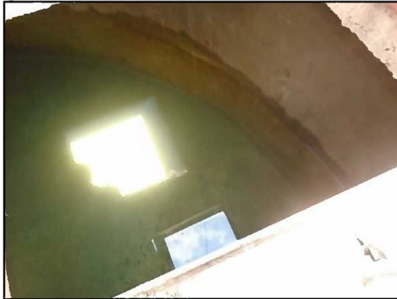
No floater valve installed
