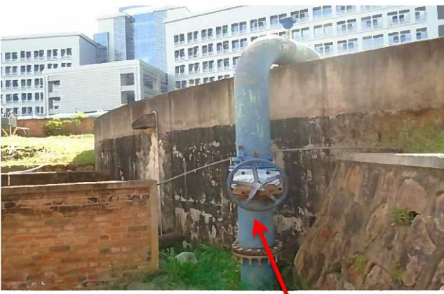
Inlet Pipe with Valve
