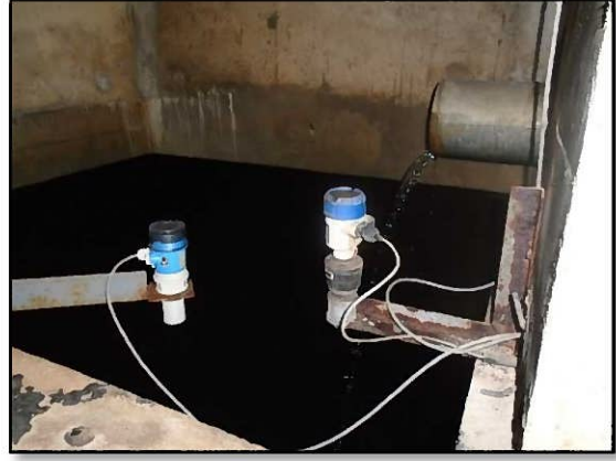
Water level indicator not working (Defective)
