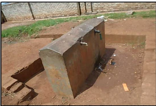
This water tap is dirty and it needs some construction works
