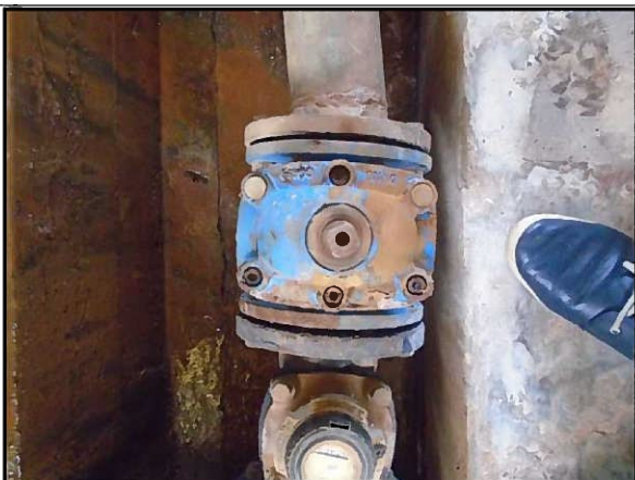
Pump outlet valve need replacement DN80
