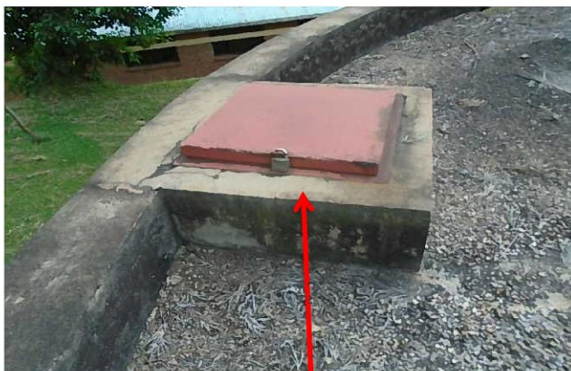
Reservoir closed (Floater is there but not fully functioning)
