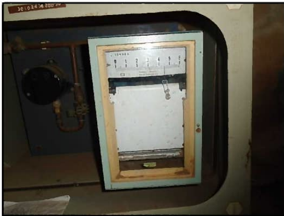
Non operational water level indicators
