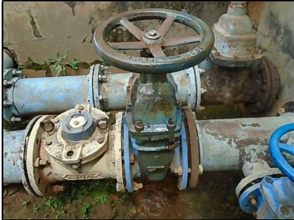
Leaking Outlet Valves
