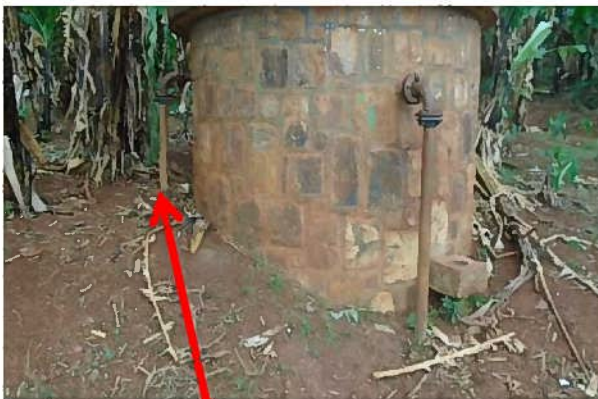
Inlet Pipe with Valve
