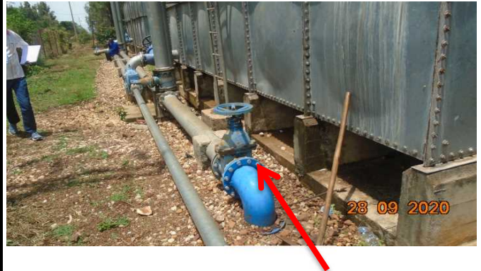
Inlet Pipe With Valve
