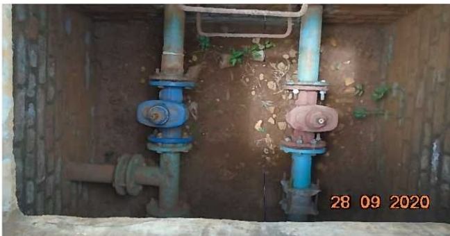
Inlet Pipe with Valve
