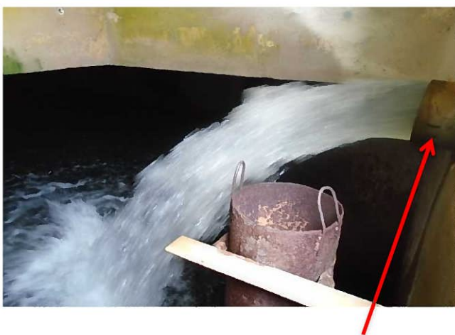
No Float Valve installed
