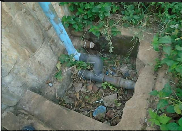
Overflow and Drain Pipe manhole need maintenance
