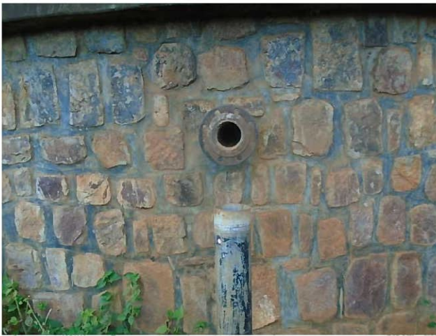
Inlet Pipe with Valve
