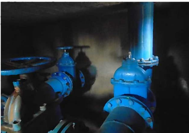
Inlet Pipe with Valve
