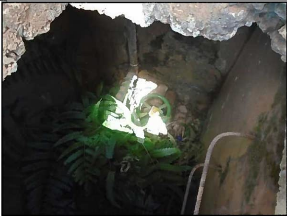
Outlet and drainage valves needed.
