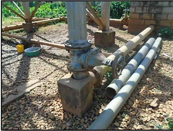
Drainage valve need replacement
