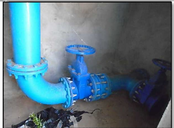
Bypass not connected
