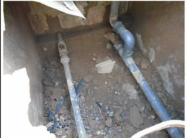
Outlet Pipe with Valve
