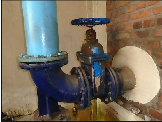
Leaking inlet Valve Res. 1
