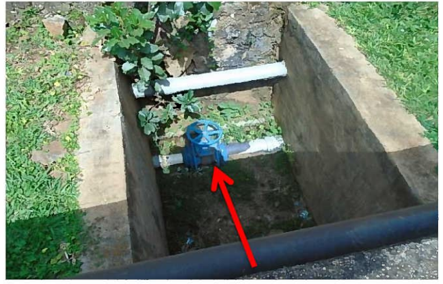
Inlet No. 4 with valve and needs to pass through a collection chamber
