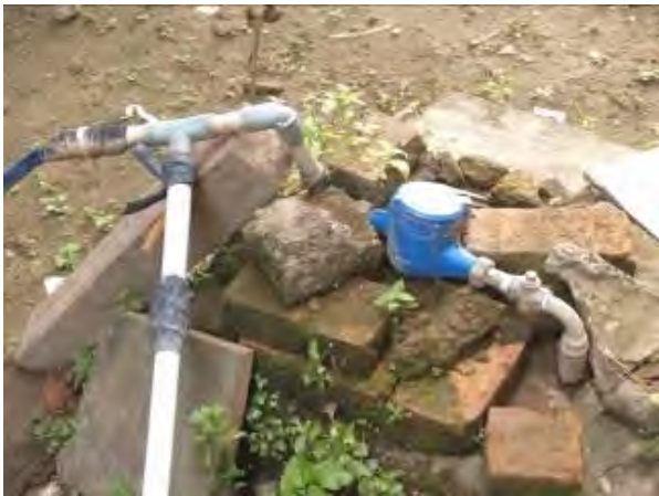
Customers aware of poor service caused by water losses will report defective connections.
