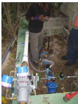
Checking accuracy of a large customer meter.
