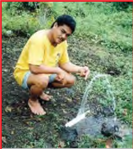
Typically more difficult to detect, service connection leaks result in significant water losses.
