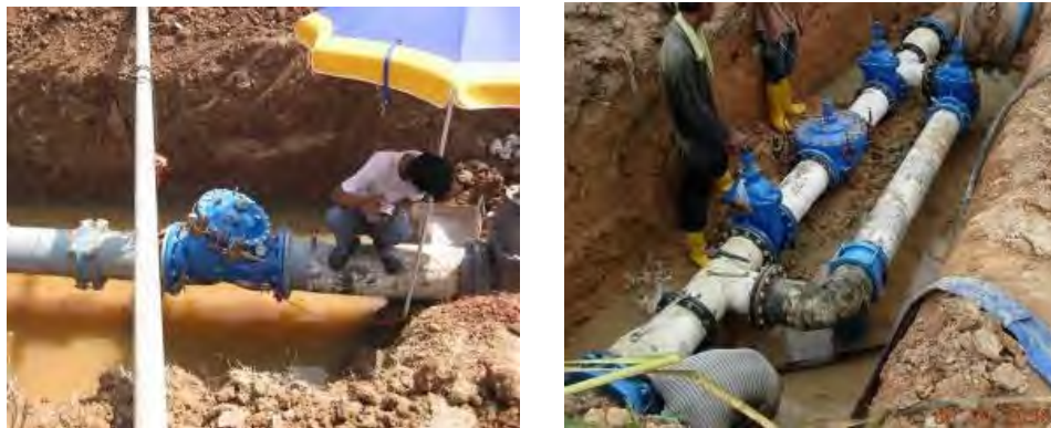
PRVs installed in meter chambers.
