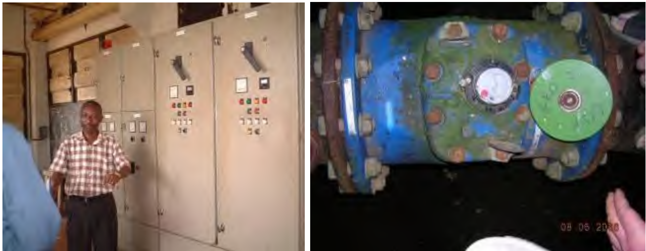
Water utility managers need to accurately measure water produced from the treatment facility. Total water produced is a key input for the water balance.
