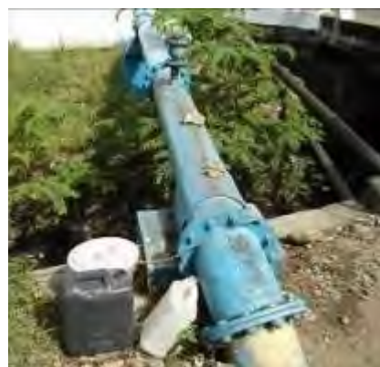
Water theft can occur from large pipes as well as from household water connections.
