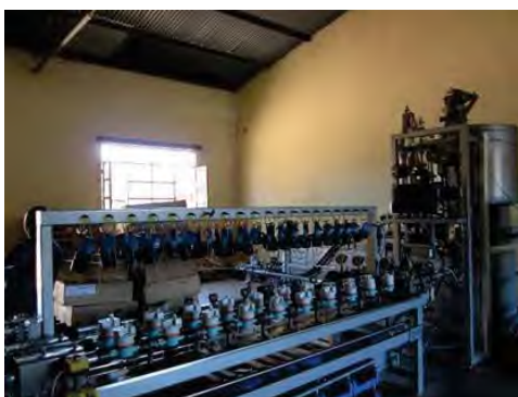
WASAC Meter Test Laboratory
