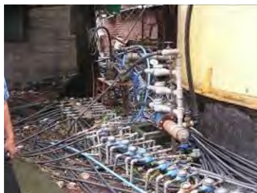
Improper meter installation leads to inaccurate data and billing errors. Meter readers in the pictured situation will find it difficult to determine which meter belongs to which property.
