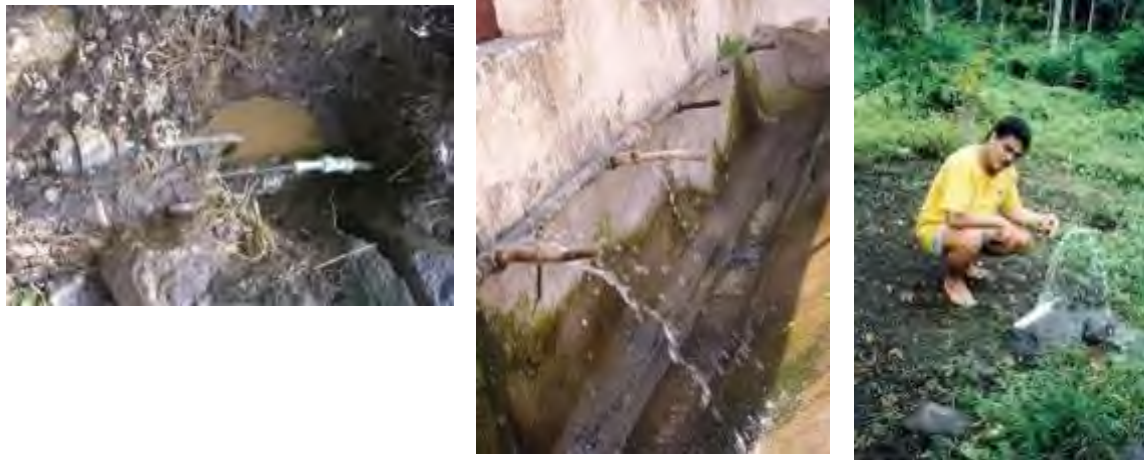
Typically more difficult to detect, service connection leaks result in significant water losses.
