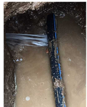
Water leakage from a HDPE pipe
