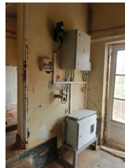
Datalogger and UPS in Pumping Station
