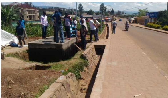
Manhole for Flowmeter in Pilot Area 1
