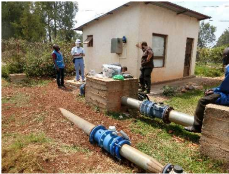
Data Transmission Facility for Monitoring System
