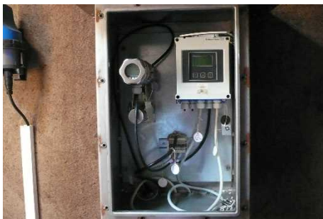
Transmitters of Flow Meter and Pressure Meter
