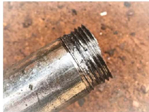
Fig.28 Screwed pipe by bad condition die
