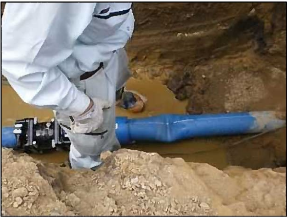
Condition after compression
