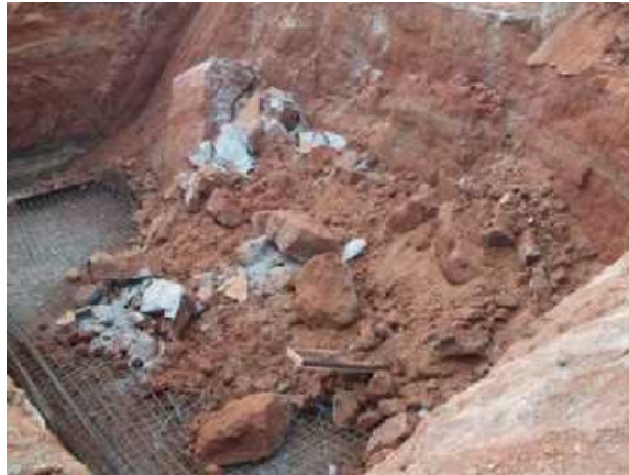
Fig.17 Soil wall collapse
