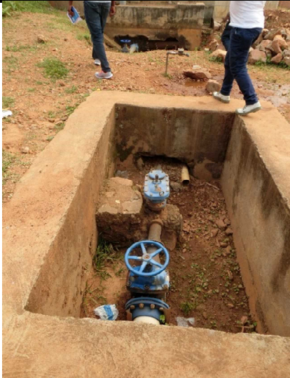
Inlet Pipe with Valve
