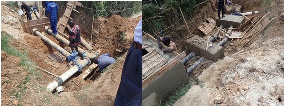
Preparation for the casting of protective concrete Valve assembly chamber and protective concrete
