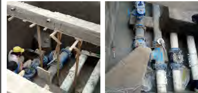
Finishing by mortar coating to the wall and finishing of pavement photos
