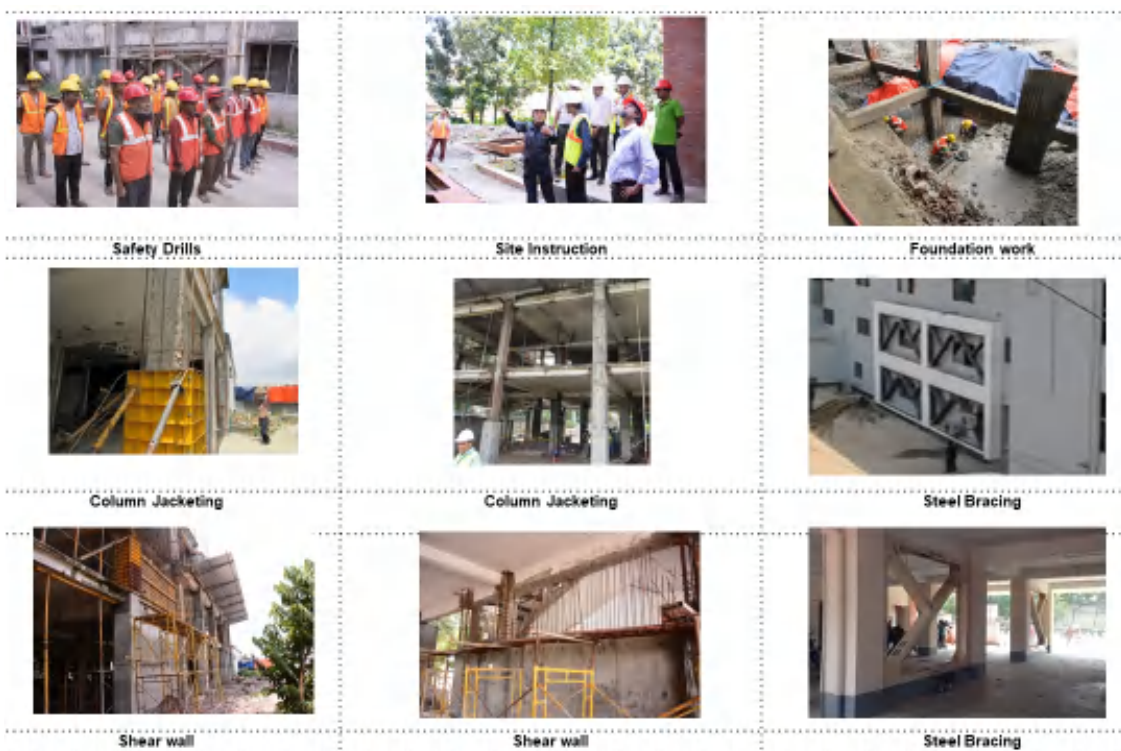
Seismic Retrofitting Works at Tejgaon Fire Station, DK Knit wear Co., Smart Knit Co.
